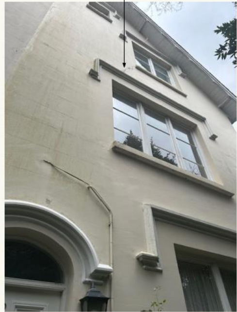
Cracks in the stucco finish on front elevation
