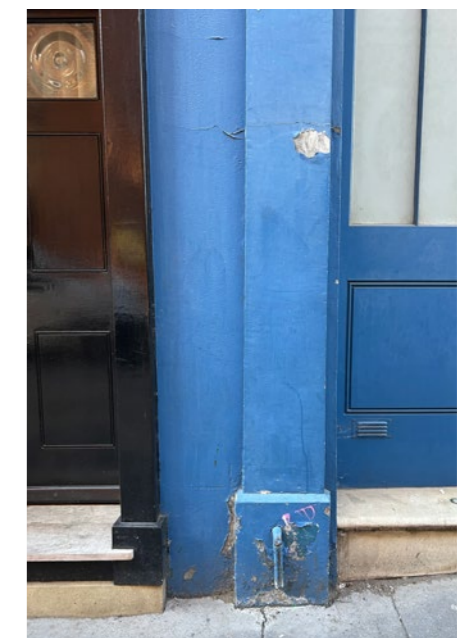
Repair works required to the front shop frontage
