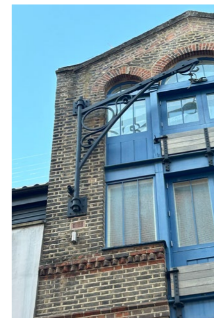
Loading crane and platform with stainless steel wall light underneath
