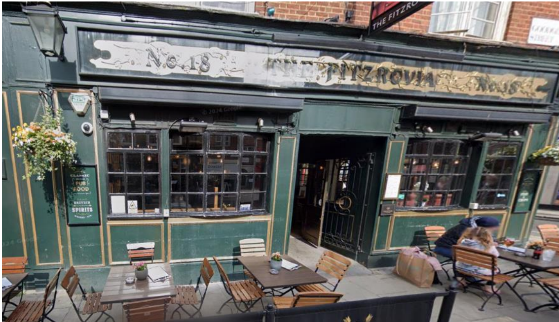
Heaters on The Fitzrovia Public House
