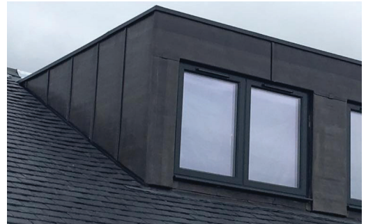
Precedent images for lead clad dormer construction in a natural slate roof
