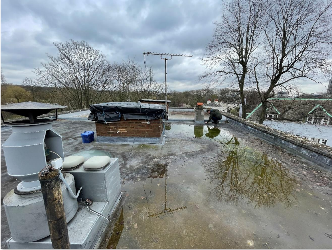
Photograph 1 – Water pooling on roof and tarpaulin cover to tank roof
