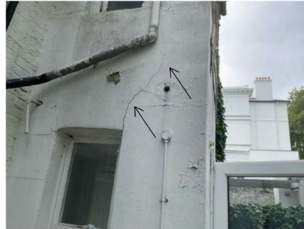
Cracking to the left side of projection heading diagonally above and below side window
