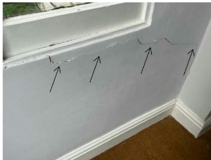
Cracking noted beneath the rear left side hallway window
