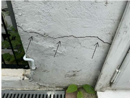
Cracking to the left side of rear external door
