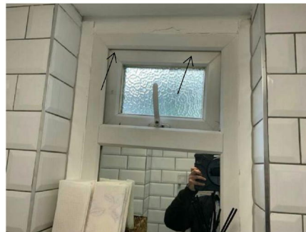
Distortions noted to the rear left WC window
