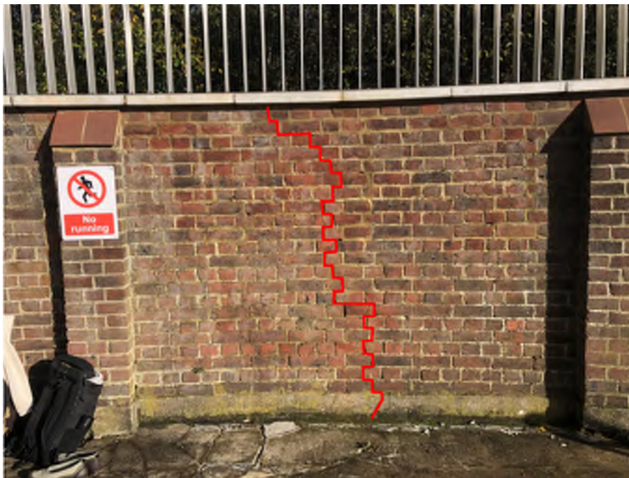
Figure 05 – Typical vertical crack on the south west elevation of the wall (red line indicates location of crack).
