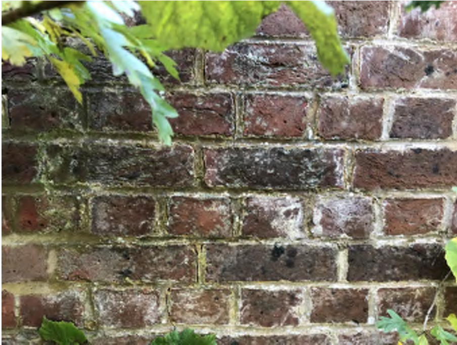
Figure 06 – Typical vertical crack on north east elevation of the wall.
