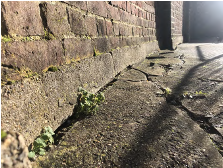
Figure 07 – Typical horizontal crack along the base of the wall showing uplift of concrete sections.
