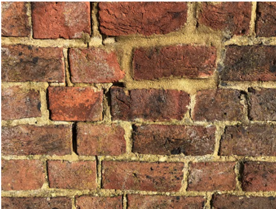
Figure 04 – Representative area of south west elevation showing the relatively good condition of the bricks and variable age and condition of the pointing mortar.
