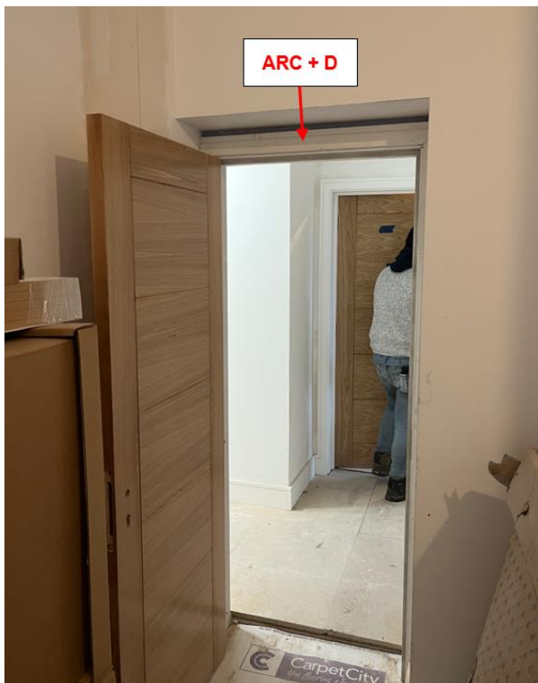
Unauthorised party wall breach, unauthorised door architraves ( ARC ) and modern door ( D ) too.
