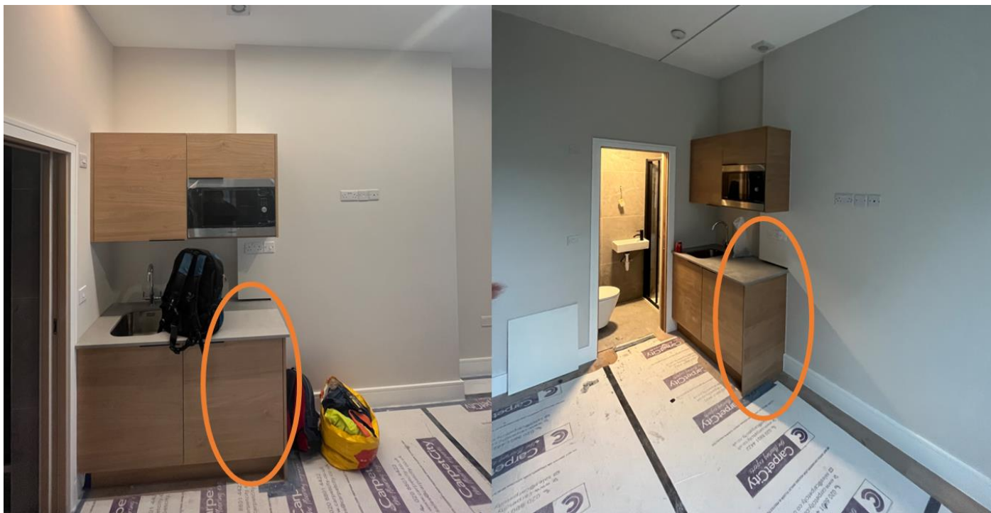
Ground floor [left] & first floor [right]: Damaged chimney breasts (circled in orange).
