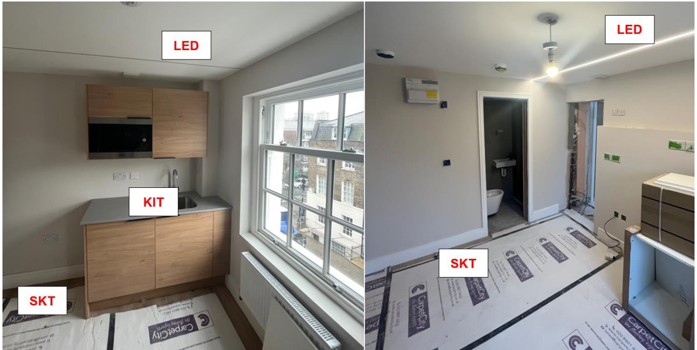
front room [left] and rear room [right]: Unauthorised door architraves ( ARC ), skirting boards ( SKT ), modern doors ( D ), MDF floorboards ( FB ), kitchenettes ( KIT ), recessed LED track lighting ( LED ).
