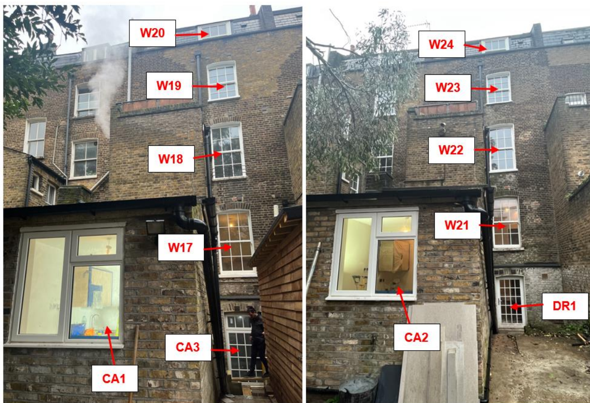
No.18 [left] & 20 [right]: EIGHT unauthorised laminated timber/composite sash windows (W17 - W24), TWO unauthorised laminated timber/composite casement windows (CA1 & CA2), ONE unauthorised laminated timber/composite top-hung casement window (CA3), ONE unauthorised laminated timber/composite door (DR1) - basement to third floor levels.
