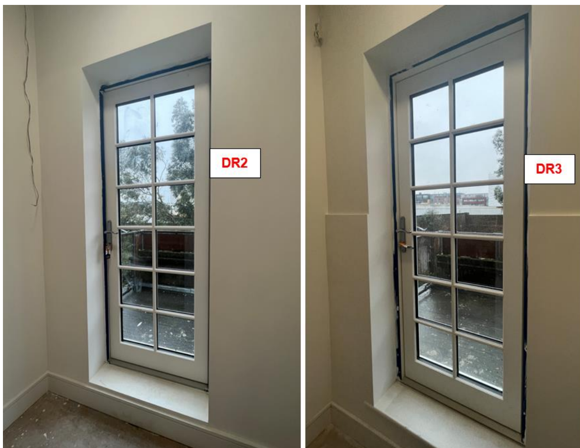
No.18 [left] & 20 [right]: TWO unauthorised laminated timber/composite doors ( DR2 & DR3 ).
