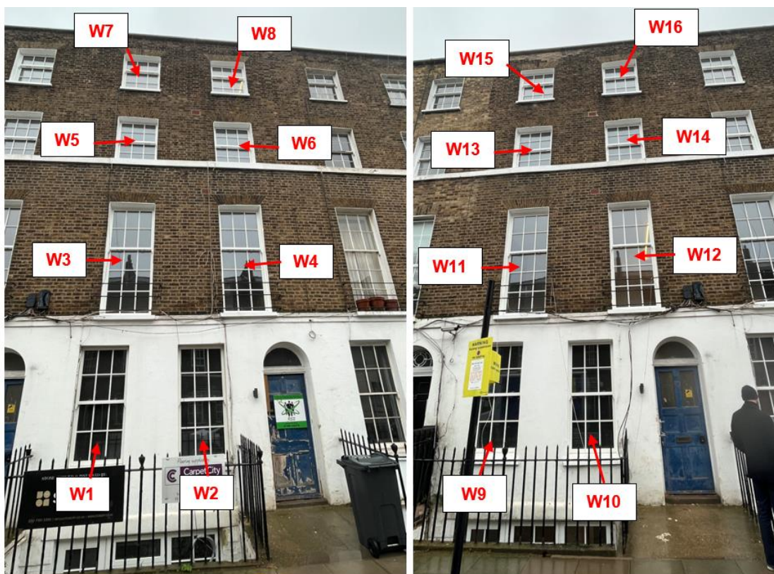
No.18 [left] and 20 [right] – SIXTEEN unauthorised laminated timber/composite sash windows (W1 - W16) - ground to third floor levels.
