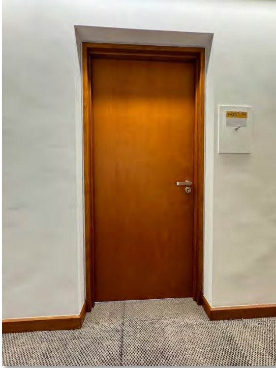
New FD30 flush panel door, stained finished to match refurbished retained door frames, architrave & skirting
