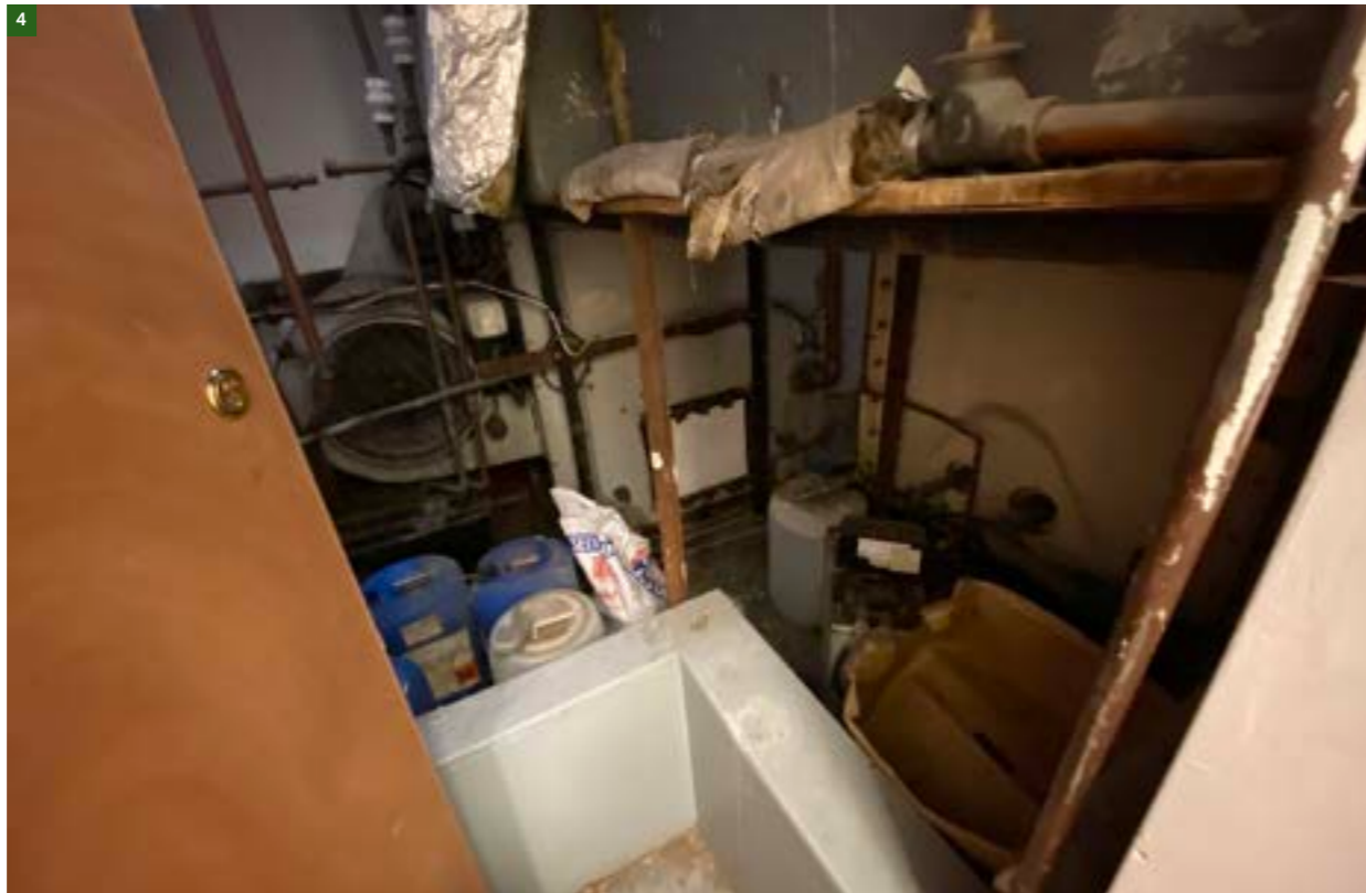
Figure 30. Fourth floor plant room in 46 BS.
