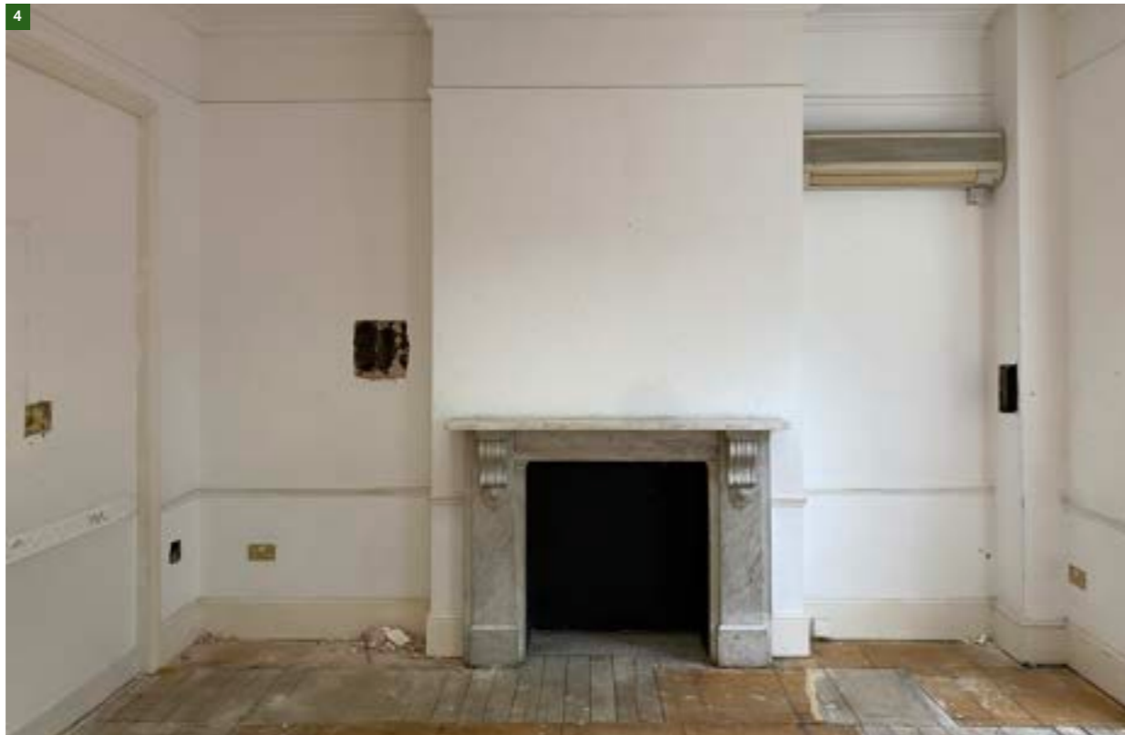
Figure 25. Existing fireplace, wall mounted FCU and in filled opening between front and back rooms in 47 BS.
