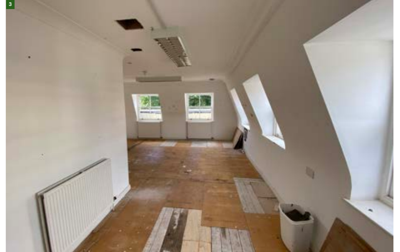
Figure 29. 46 BS office space with plant room on left.
