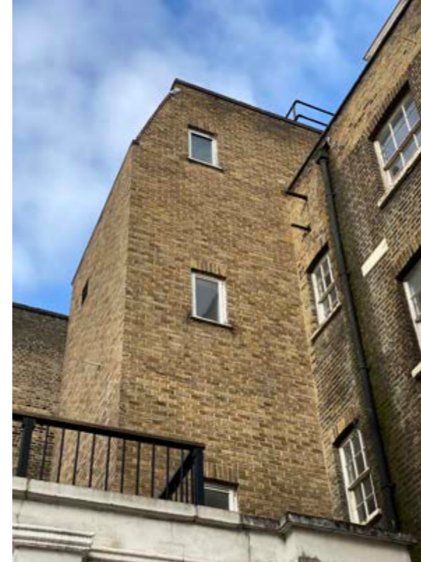
Figure 6. Rear of 20-21 showing facade condition and 1970s lift and WC core.
