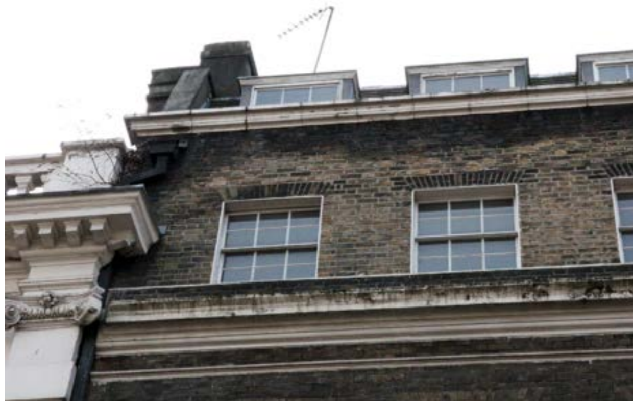
Figure 4. Existing photo of 20-21 showing façade condition.
