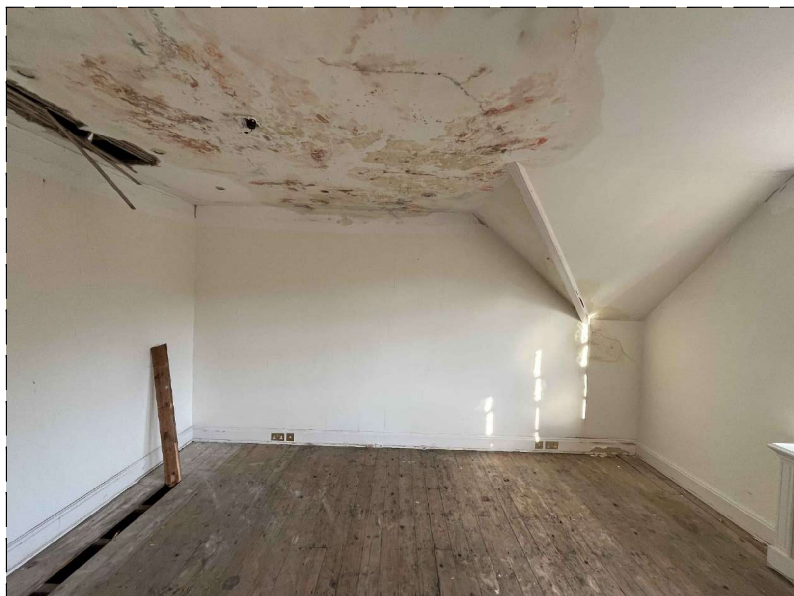
Image 4 - View of 2nd floor ceiling damages from roof leaks
