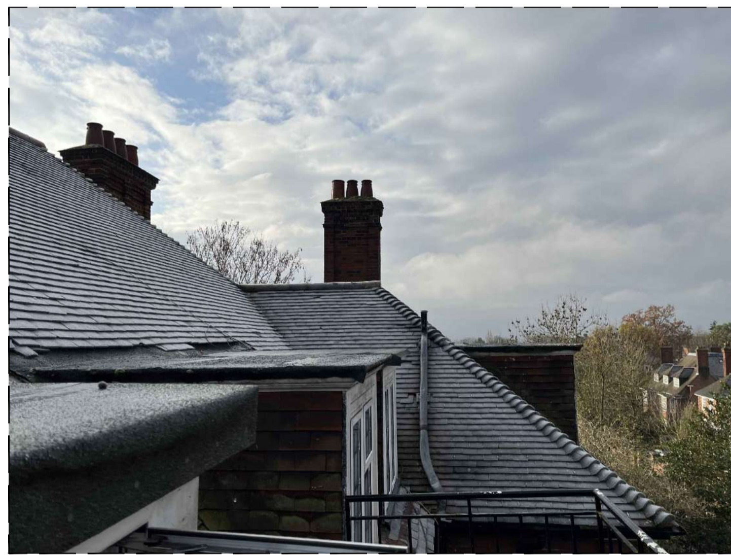
Image 4 - View of state of felt & clay roof
