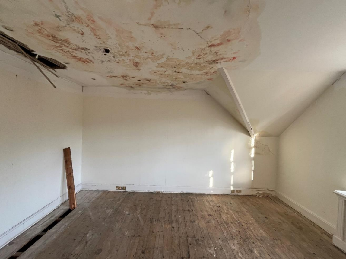
Figure 18: Water damage to lath and plaster ceiling on second floor.
