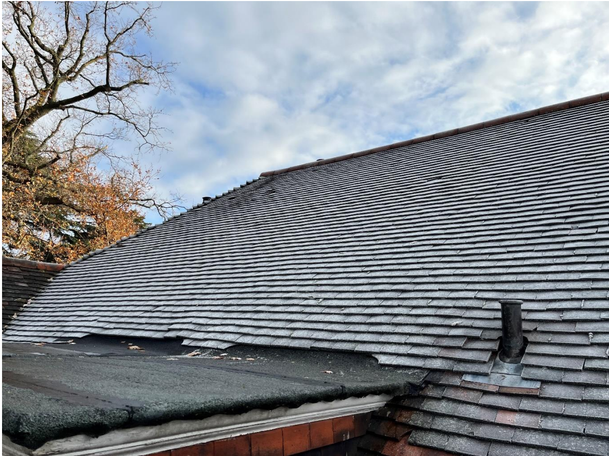
Figure 7: Front slope looking northeast. Note the junction of the tiles with the felt roof of a front dormer, and the missing string of clay tiles. There are clearly some patches in the roof with missing/ broken tiles that are in need of attention. The felt roof on the dormers are to be replaced with lead – a more durable, historically appropriate material for a dormer.
