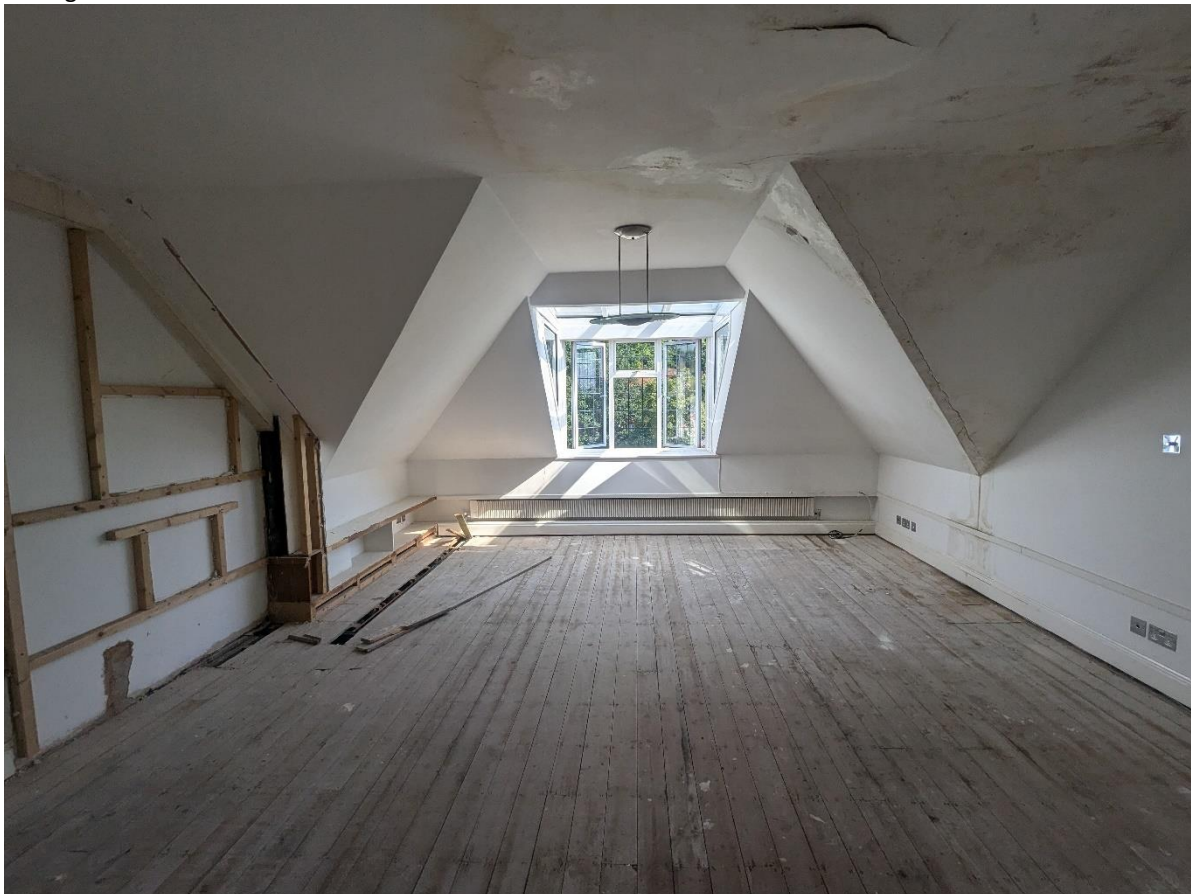
Figure 17: Water damage to the ceiling and dormer alcove.
