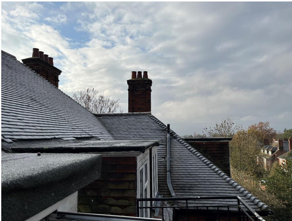
Figure 9: View of the front roof slope from the central balcony looking to the southern wing of the house. There are four dormers in this view with tile hanging, flat felt topped dormers and obtrusive vent on the projecting south wing. The condition of the chimney stacks will be reviewed during the roof works.
