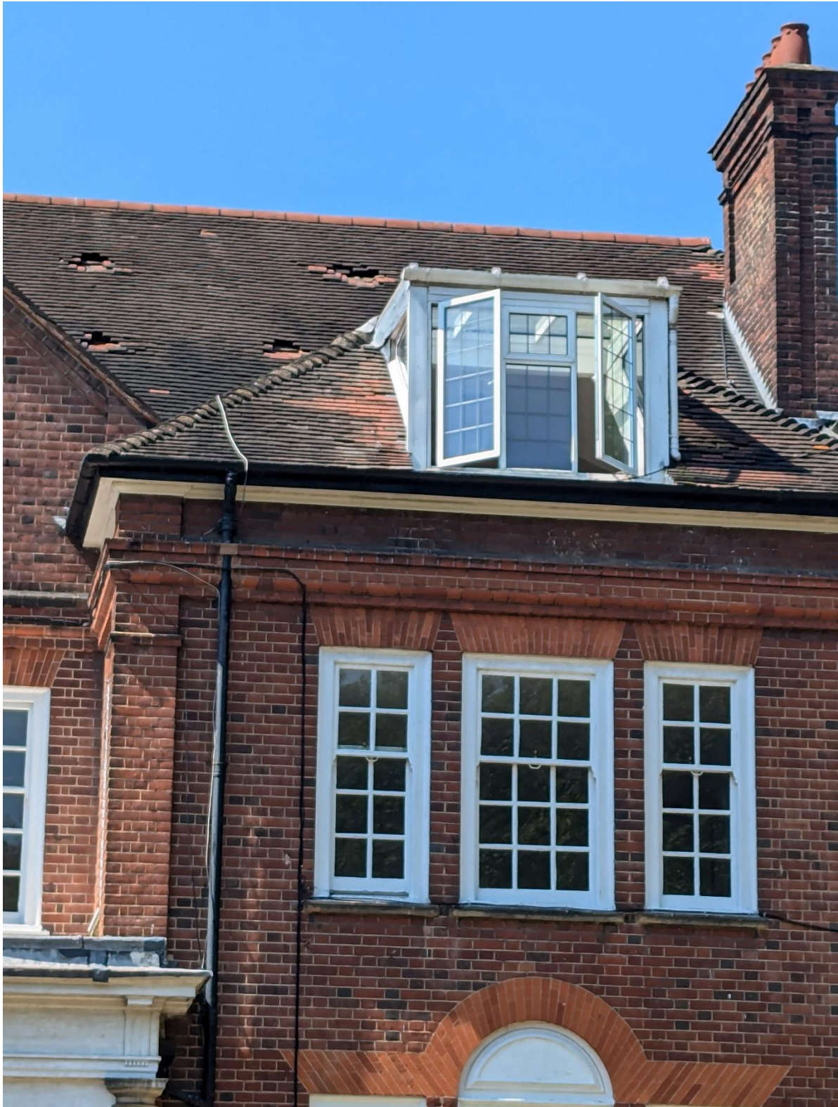
Figure 12: View of the rear roof slope. It is clear in this image the holes in the roof and the patch repairs around the glazed dormer. These holes are the source of the water ingress and associative damage throughout the property.
