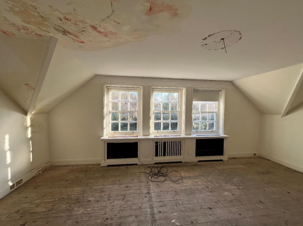
Figure 19: Water damage to lath and plaster ceiling on second floor.
