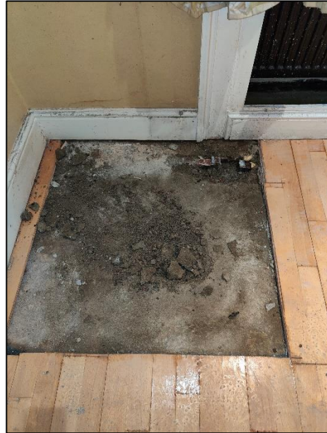
LOWER GROUND FLOOR TP1 75mm sand cement screed on 250mm thick concrete slab
