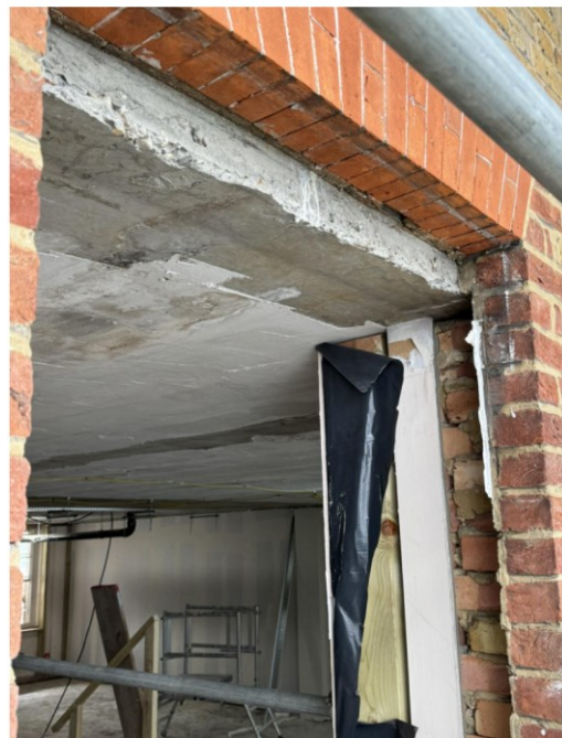
Figure 2 & 3: Existing concrete frame restricting the
