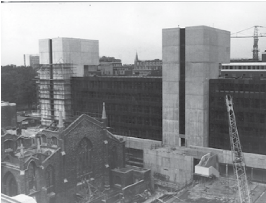
Fig. 11: No. 20 Bedford Way under construction, mid-1970s, viewed from Thornhaugh Street, facing north Institute of Education Archive
