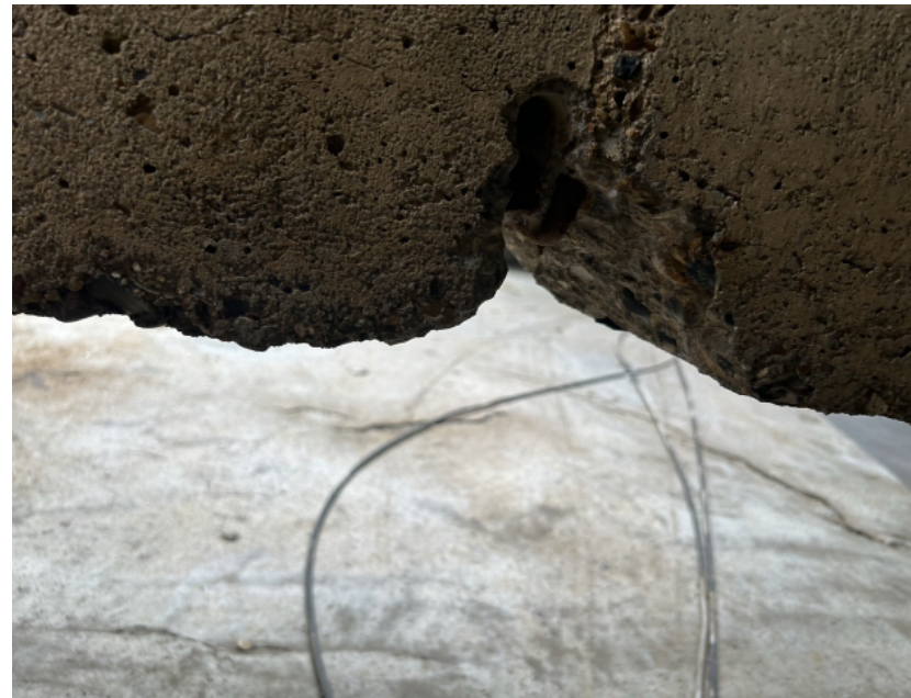
Image showing spalling of RC beam supporting existing roof plant
