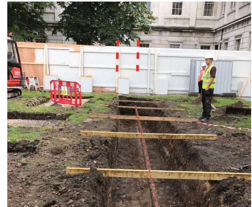
Existing gas main
