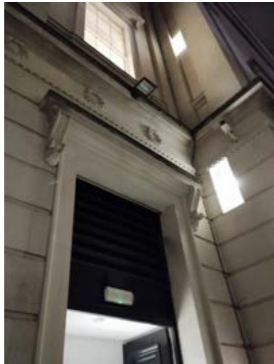
Some entrances had additional emergency bulkheads
