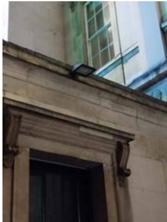
Facade mounted flood lights, presumably for emergency escape
