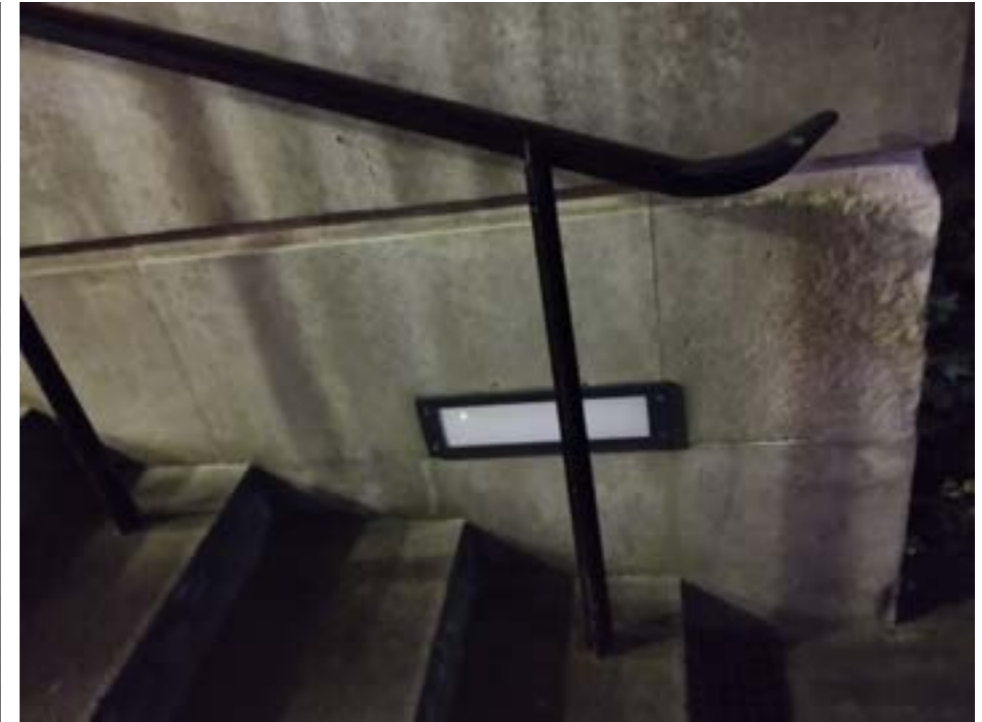
Wall mounted luminaires, presumably for emergency escape
