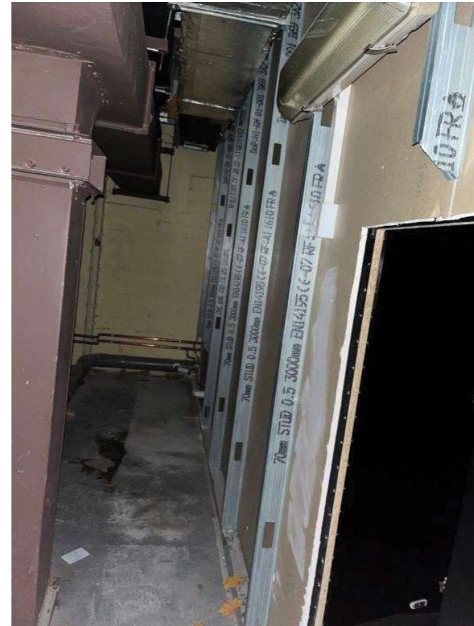
The above photograph shows the space to the rear of Unit 3 at UGF level. The stud work wall to the right is part of the current arrangement of the mezzanine level of the Retail Unit. This space is currently used as a service void with access for maintenance.
