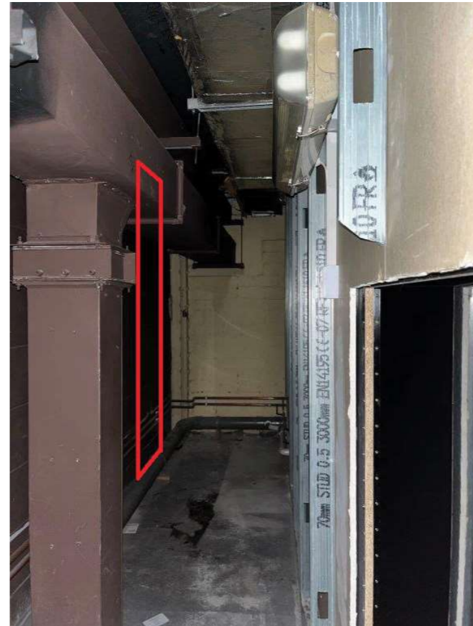
The above photograph shows the space to the rear of Unit 3 at UGF level. The red outline showing where the door is proposed to be located
