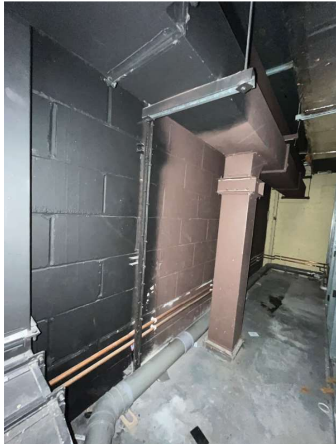
The above photograph shows the space to the rear of Unit 3 at UGF level. The MEP equipment will be modified to allow for access to the new proposed access door to be created in the block wall through to the south atrium.
