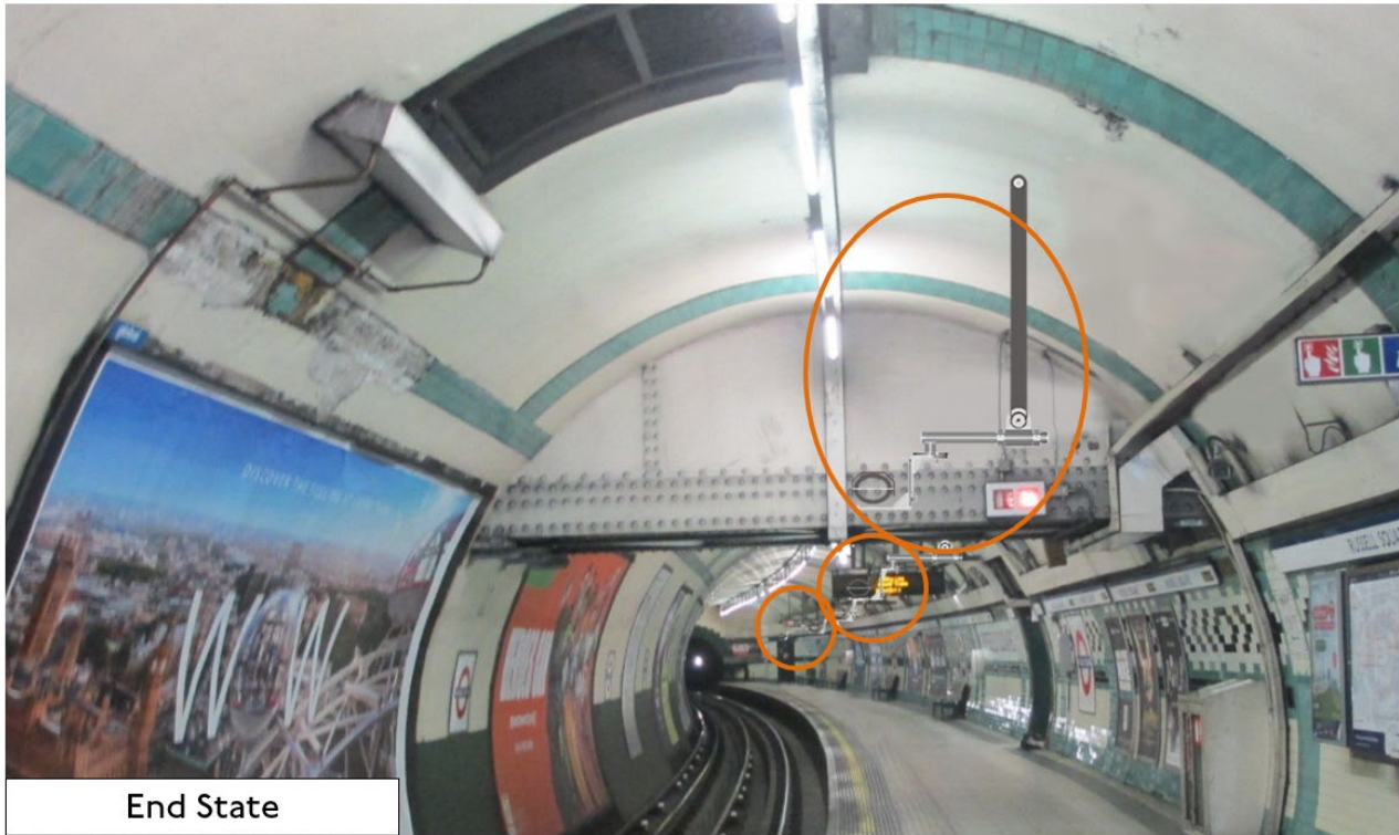
Figure 9: Platform 2 cameras during the migration phase. The existing camera is highlighted in purple, the new cameras are shown in orange.
