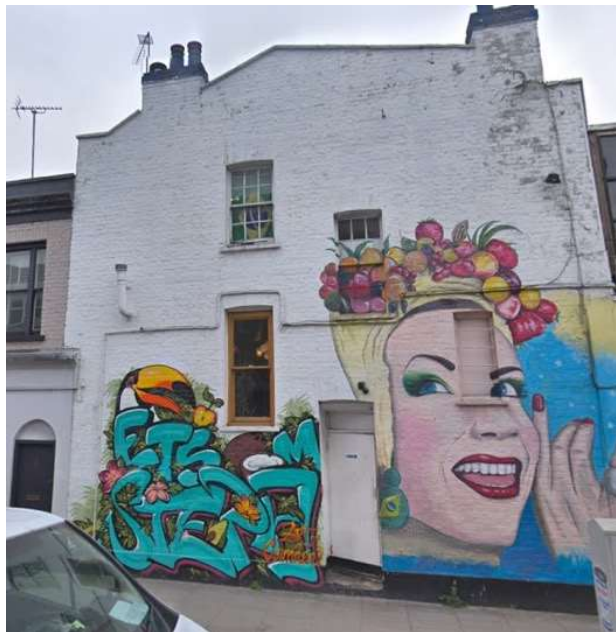
Figure 5 - Previous tagging/unauthorised painting
