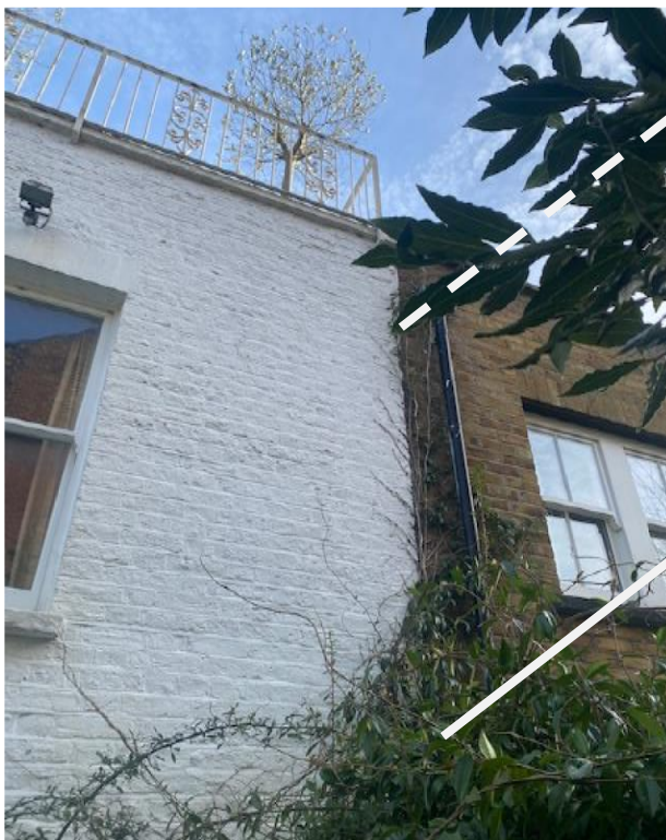
Photo 4: The existing roof terrace at the second floor level, on top of 11 Willoughby Road's existing extension would overlook the proposed roof terrace, creating an overlooking problem.
