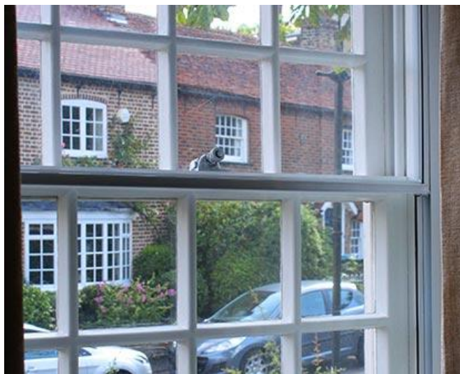
Photograph showing typical sash and secondary glazed arrangement (secondary with top and bottom opening panels)
