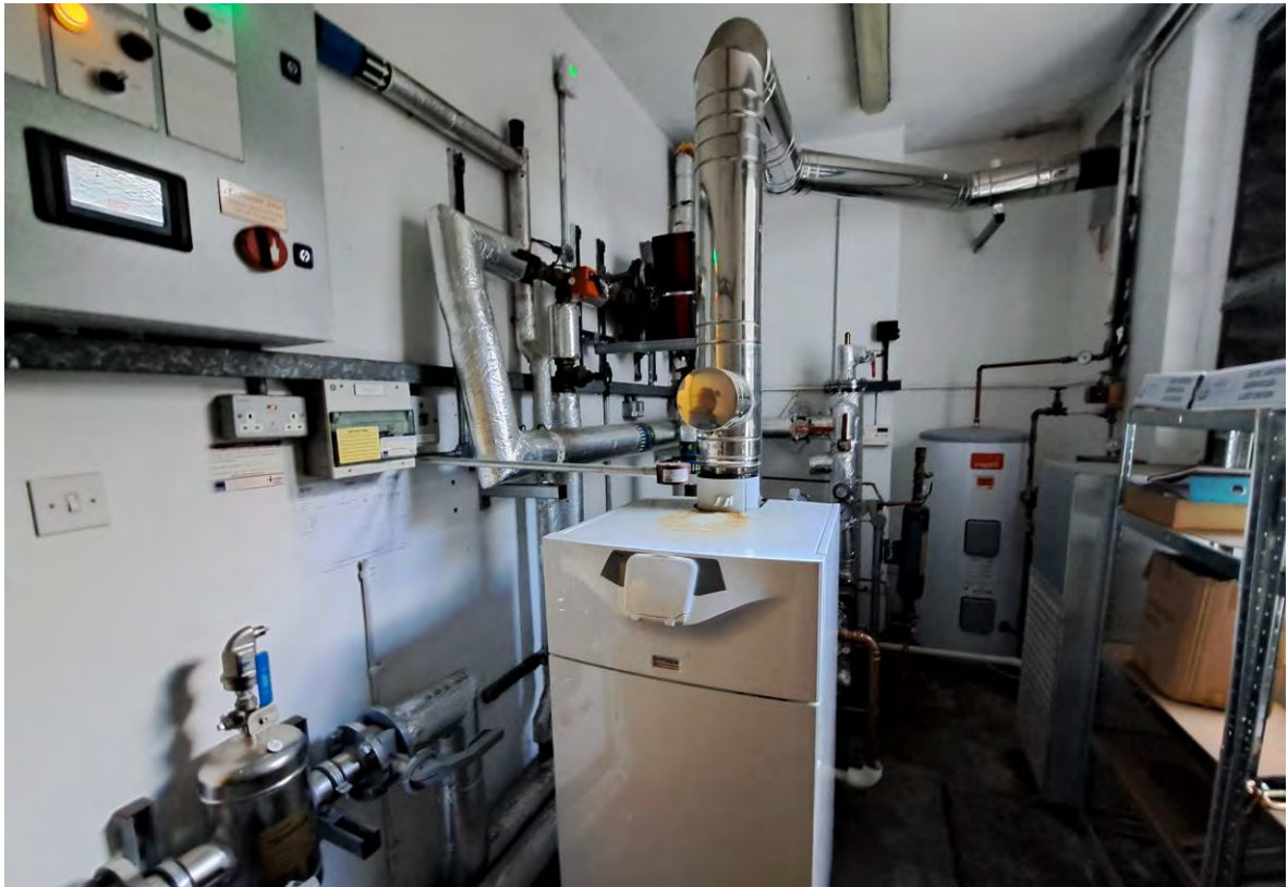
Photo 06: Boiler room on lower ground floor.
