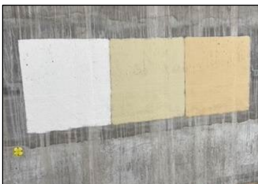
Figure 2: Proposed paint colours which were considered and discounted (chosen colour 9332 is the middle sample)
