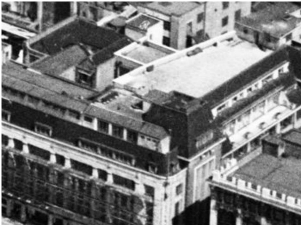
Figure 2.2: Roof of Heals Building in 1946 demonstrating (image provided by Britain from Above)
