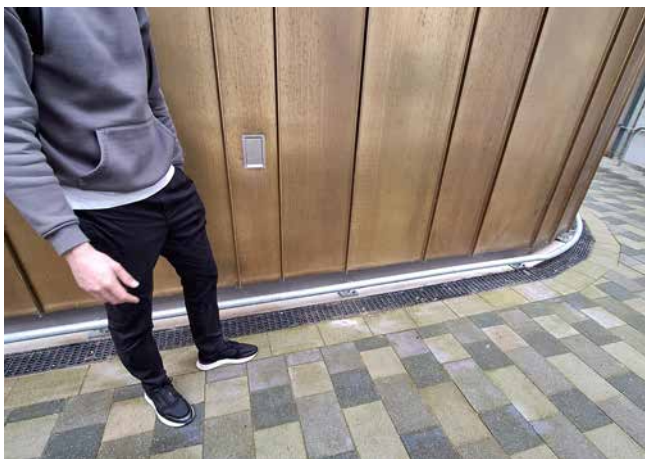
Fig. 08 Standing seam cladding to be penetrated at ground floor ceiling level (internally).
