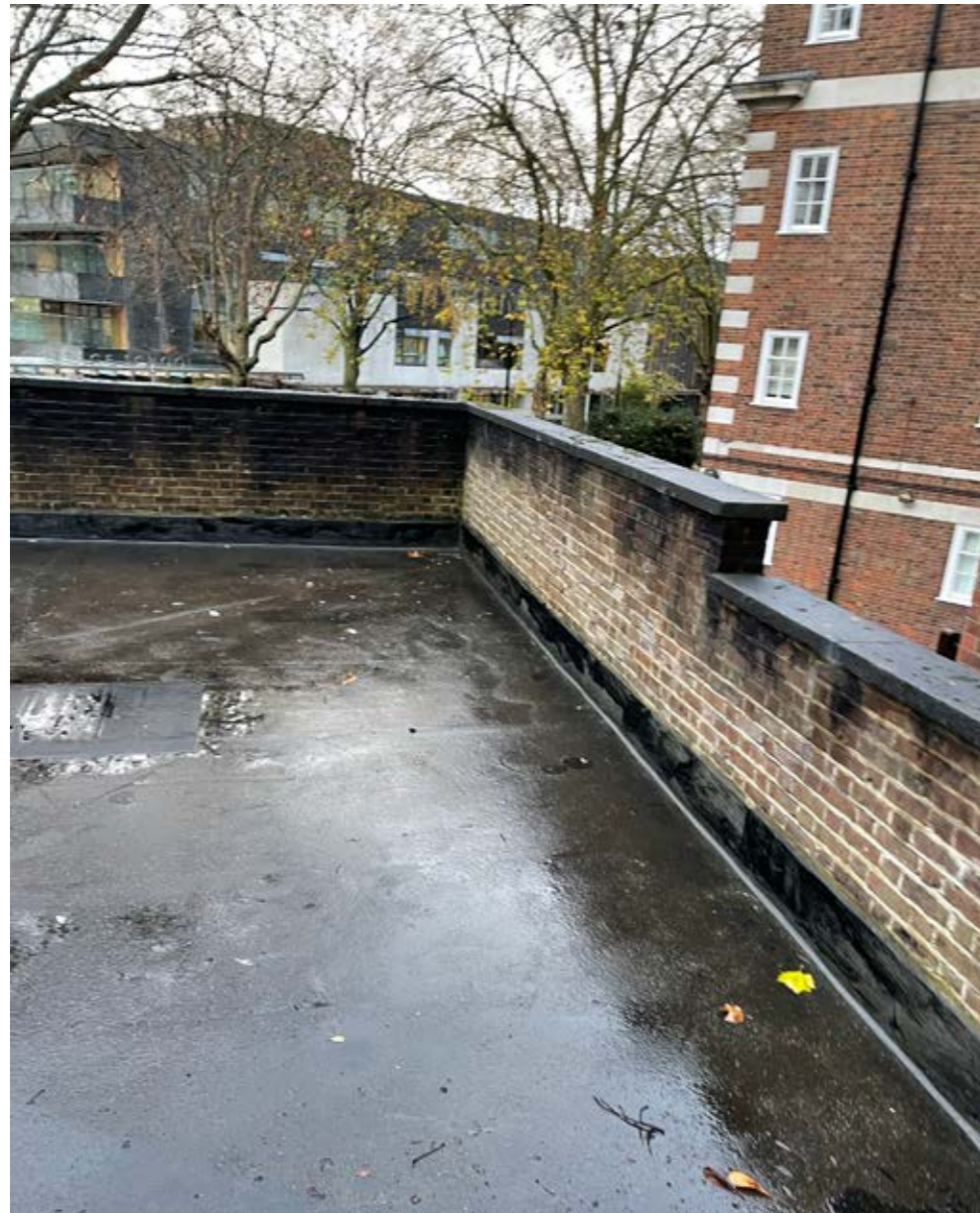
Fig 16. Looking east towards Avenue Road with a view of the existing garage roof and the associated parapet wall over with coping.
