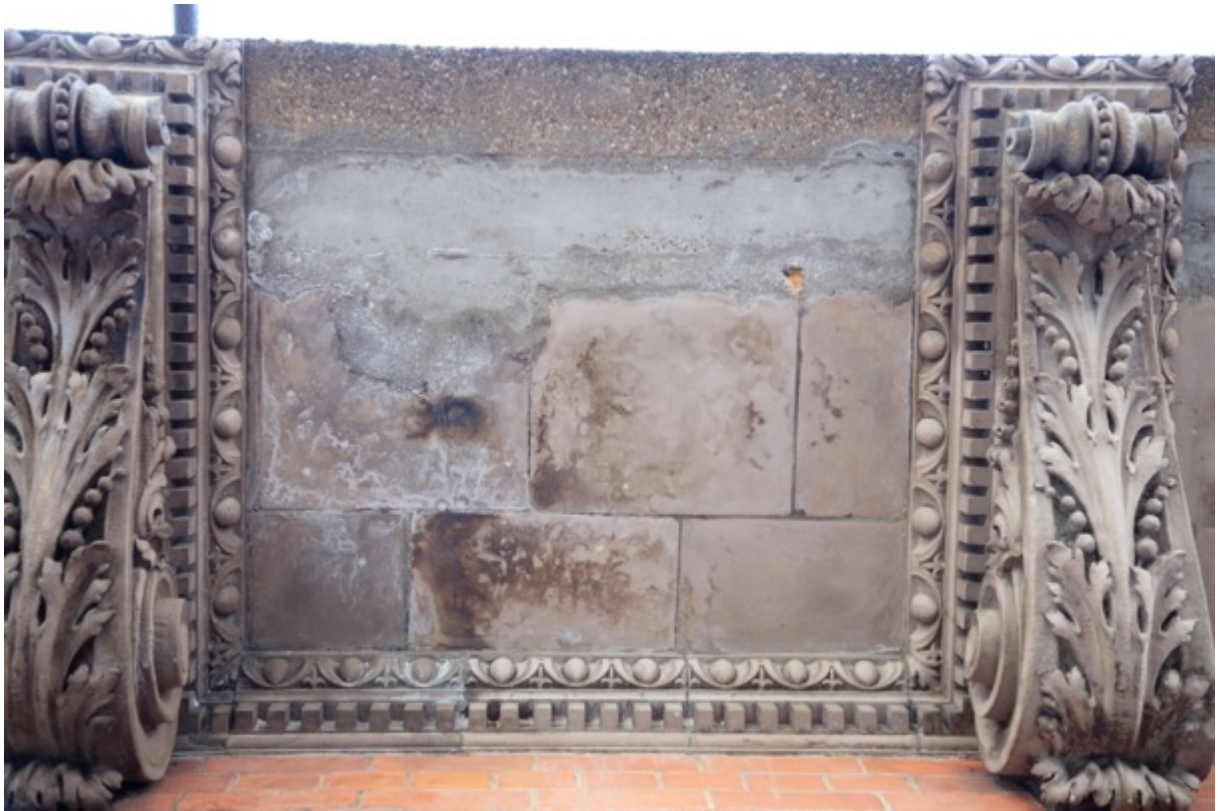
Figures 7 and 8. Two sections of the balcony soffit illustrating missing tiles along the front edge and remaining tiles with extensive damage. This condition applies to the entire soffit.
