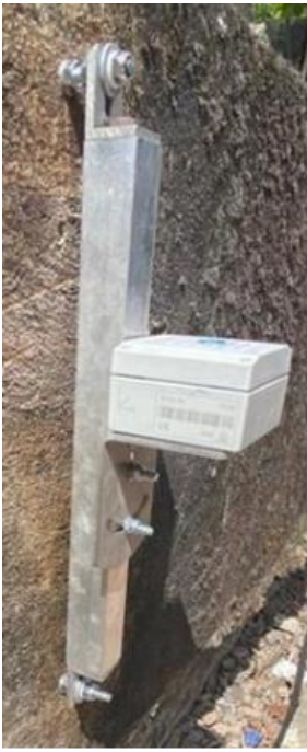
Figure 11– Example of a tiltmeter
