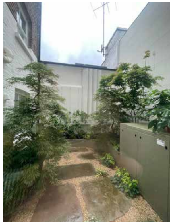
Acoustic Enclosure in situ on another Camden Project
