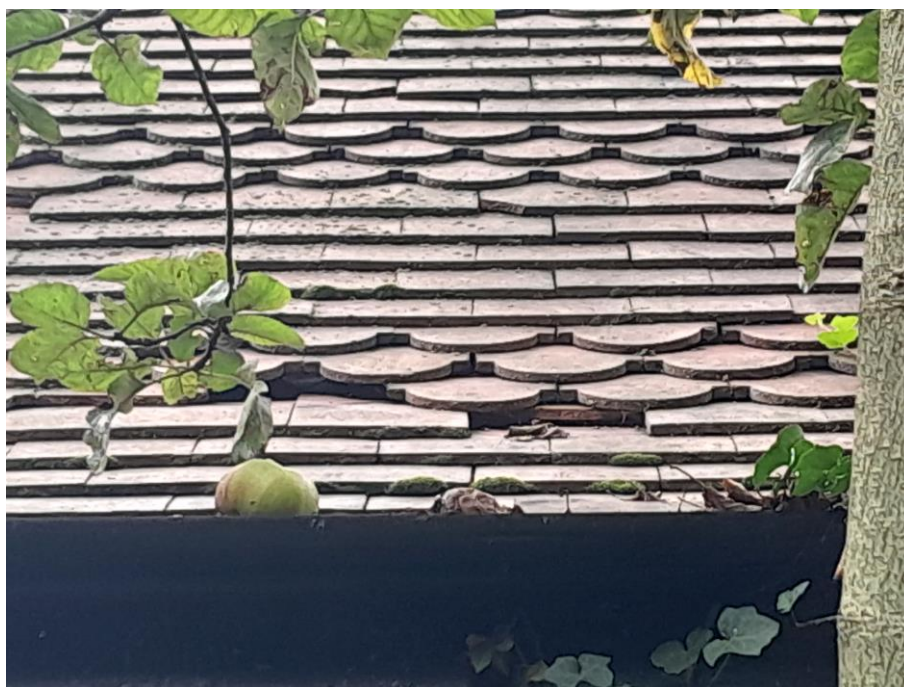
Photograph 5: Missing tiles on building B2 (Target Note 1, Figure 1)
