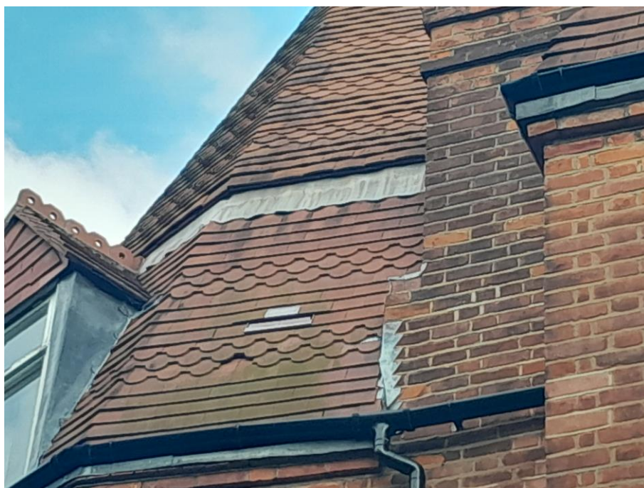
Photograph 7: Missing tiles and gaps under flashing of building B1 (Target Note 3, Figure 1)
