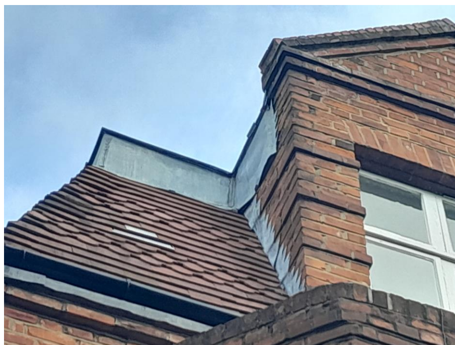
Photograph 6: Missing tiles and gaps under flashing on building B1 (Target Note 1, Figure 1)
