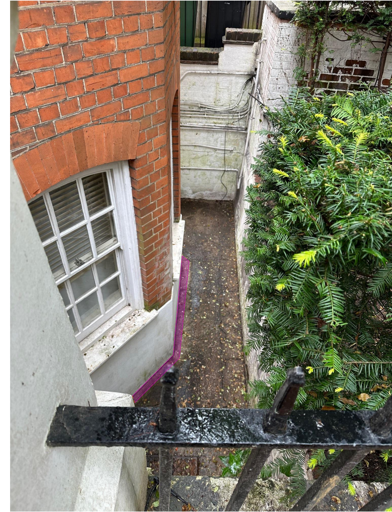
Lightwell - All plants have been removed ACO drain channel to be provided - as discussed with Hutton and Rostron - to protect the wall.
