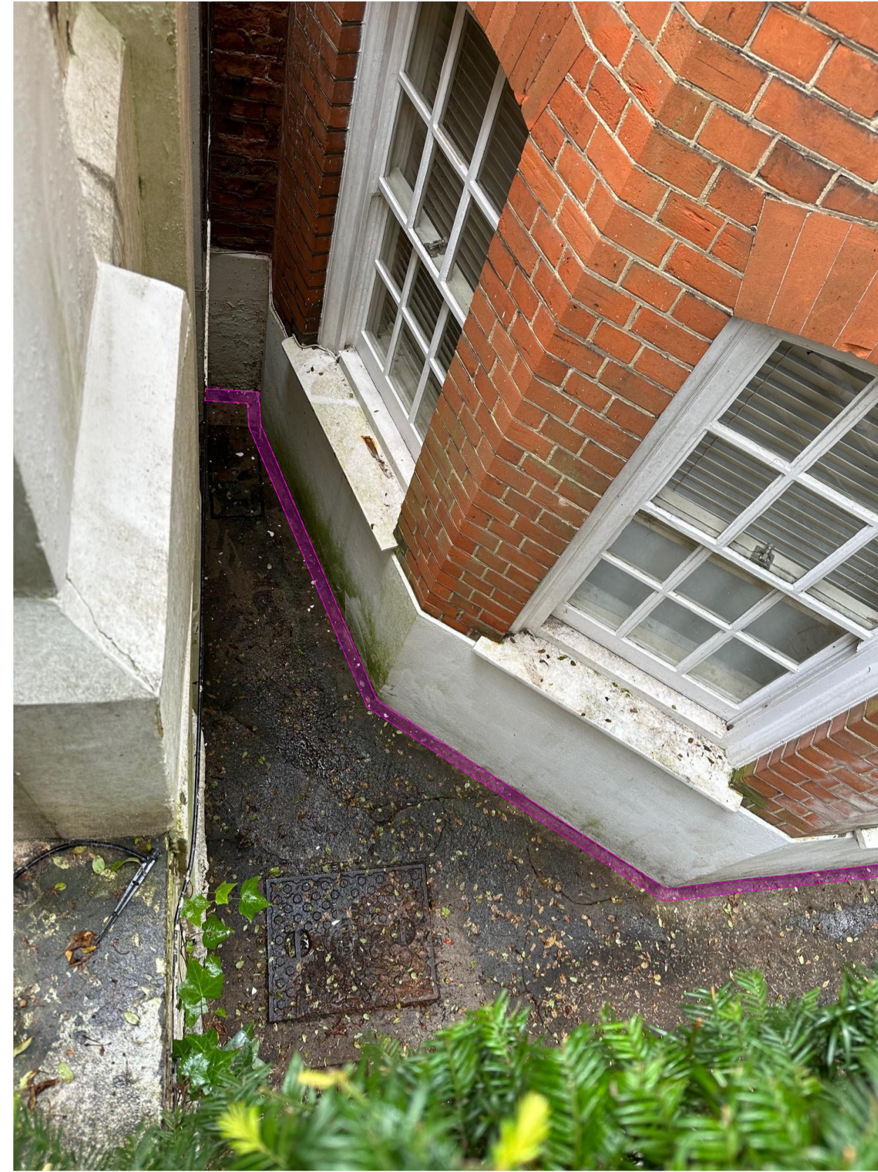
Lightwell - All plants have been removed. Manhole cover to be replaced ACO drain channel to be provided - as discussed with Hutton and Rostron - to protect the wall.
