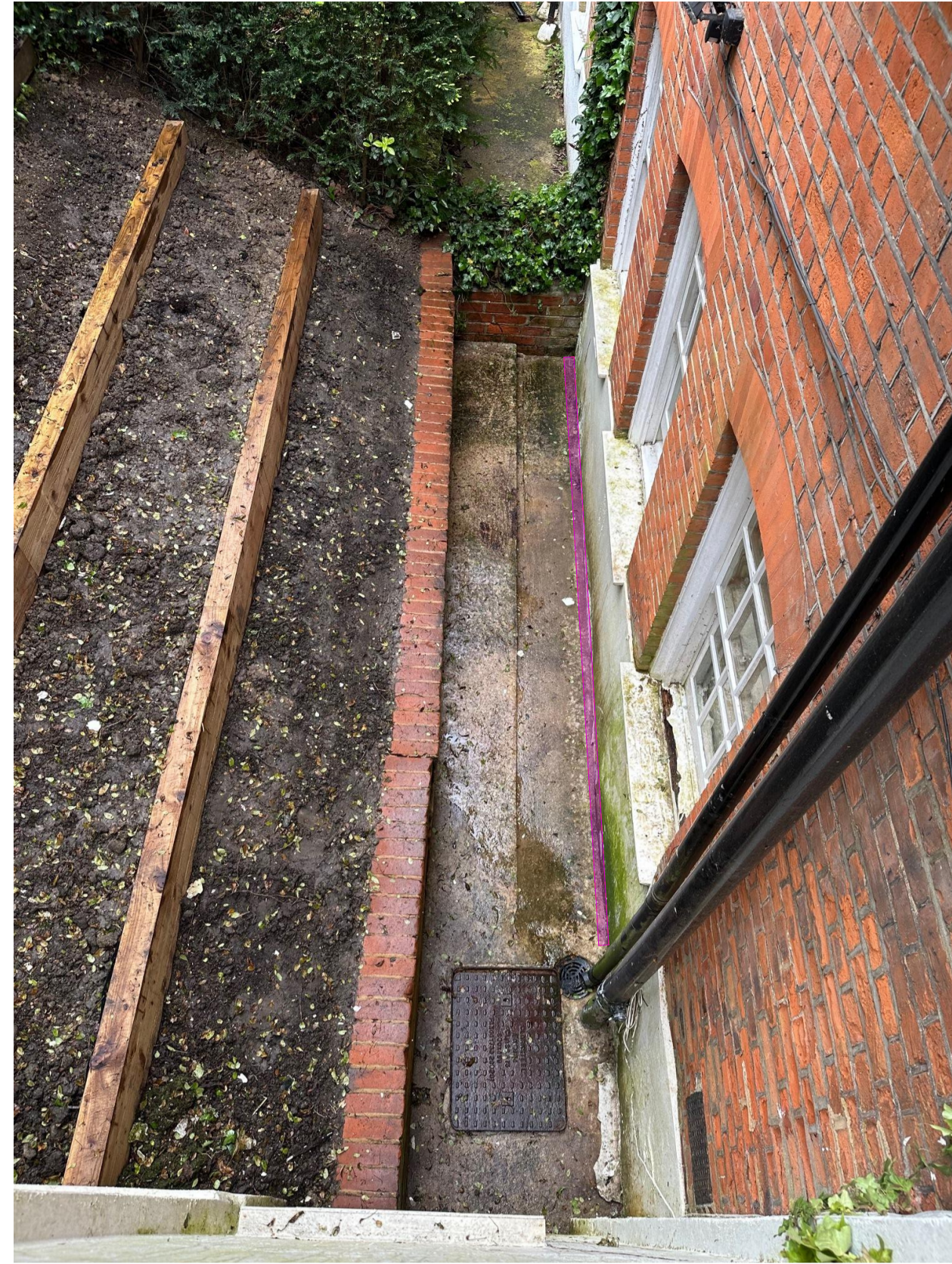
Lightwell - All plants have been removed ACO drain channel to be provided - as discussed with Hutton and Rostron - to protect the wall.
