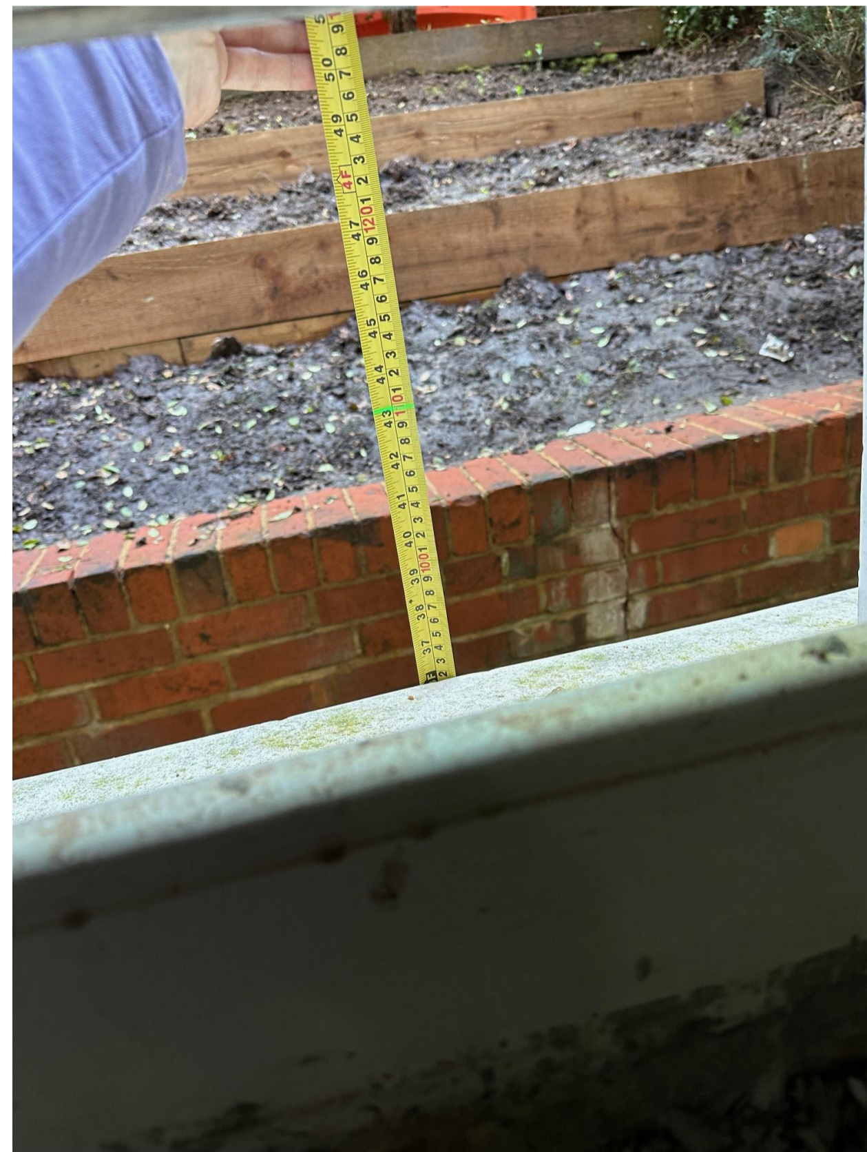
Lightwell level is higher than internal FFL, but internal build up is still missing
