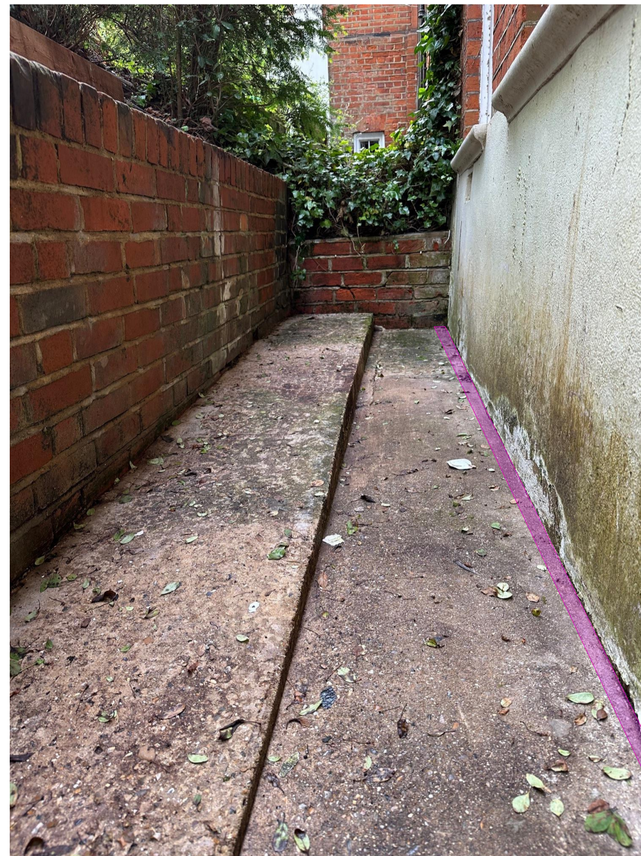
Lightwell has been cleaned ACO drain channel to be provided - as discussed with Hutton and Rostron - to protect the wall.
