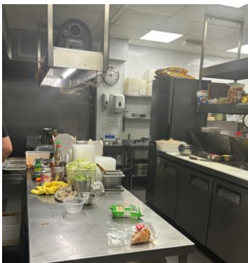
Commercial kitchen showing suspended kitchen and panel lights
