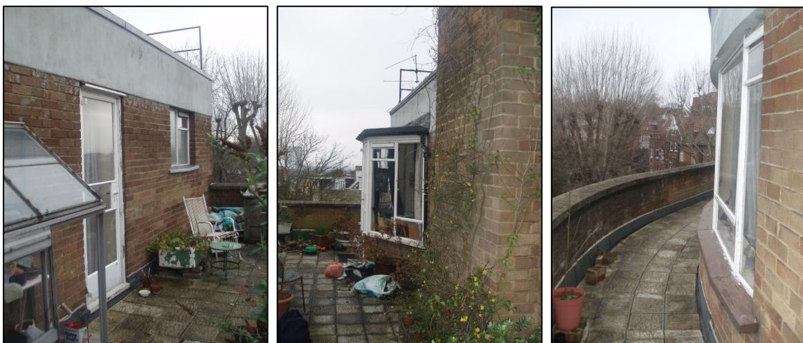
Figure 15 – Submitted photos which accompanied the 2009 application. Images show that the entire roof is in use as a terrace.
