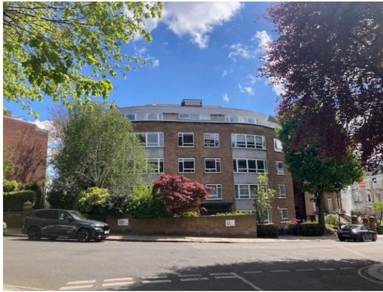
Figure 23– Photograph of balustrade as installed (note that the proposals are for a reduced amount of glass balustrading).
