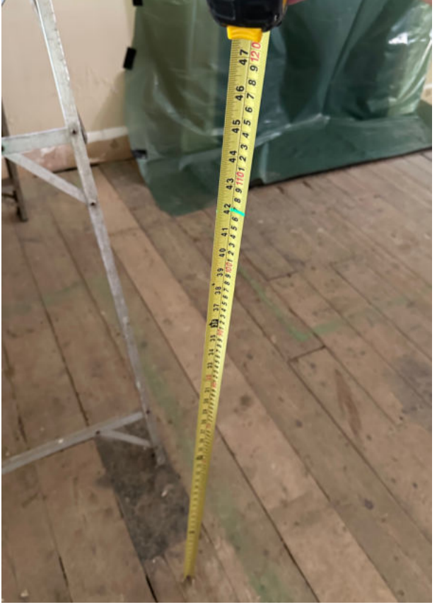
Picture 5 - Highest point of timber floor (1068mm = -46mm)
