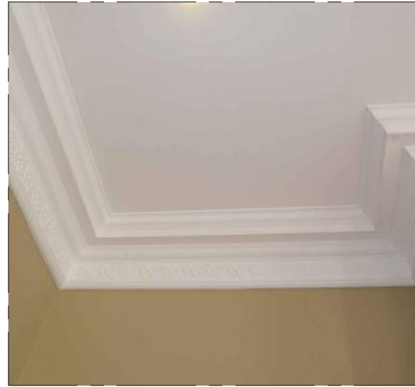
03 EXISTING CORNICE 03 - PROPOSED CORNICE TYPE B GROUND FLOOR - R02 & R03 FORMAL LIVING & DINING
