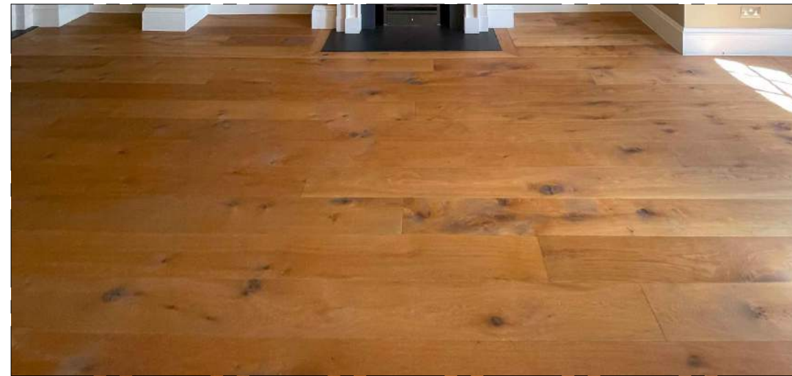
04 FLOORING 04 - TO BE REPLACED GROUND FLOOR - R02&R03 FORMAL LIVING & DINING
