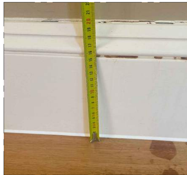
07 EXISTING SKIRTING 03 - PROPOSED SKIRTING TYPE A GROUND FLOOR - R02&R03 FORMAL LIVING & DINING
