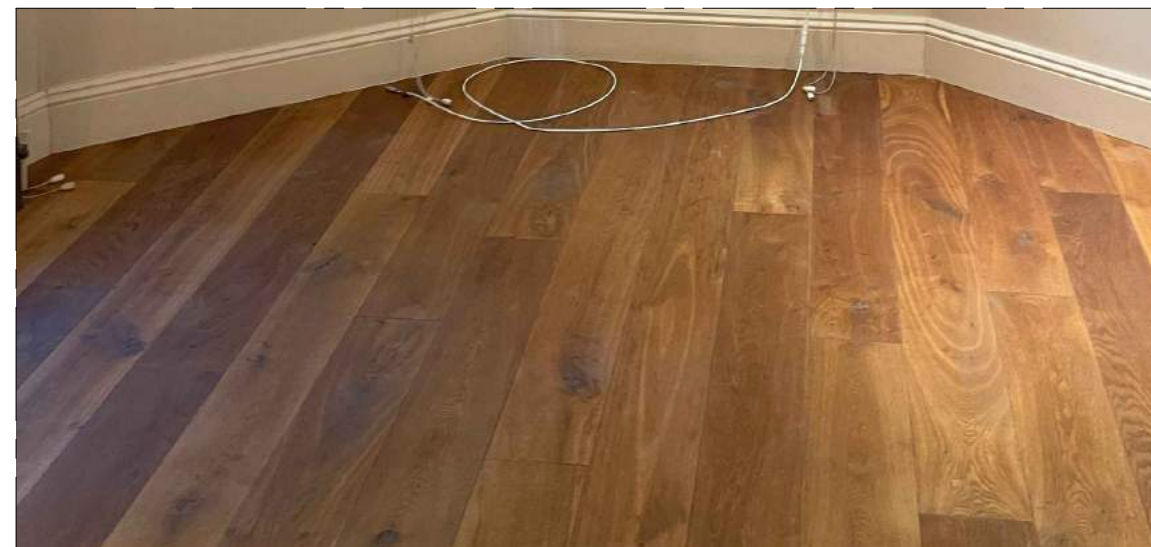
06 FLOORING 06 - TO BE REPLACED LOWER GROUND FLOOR - R14 BEDROOM 03
