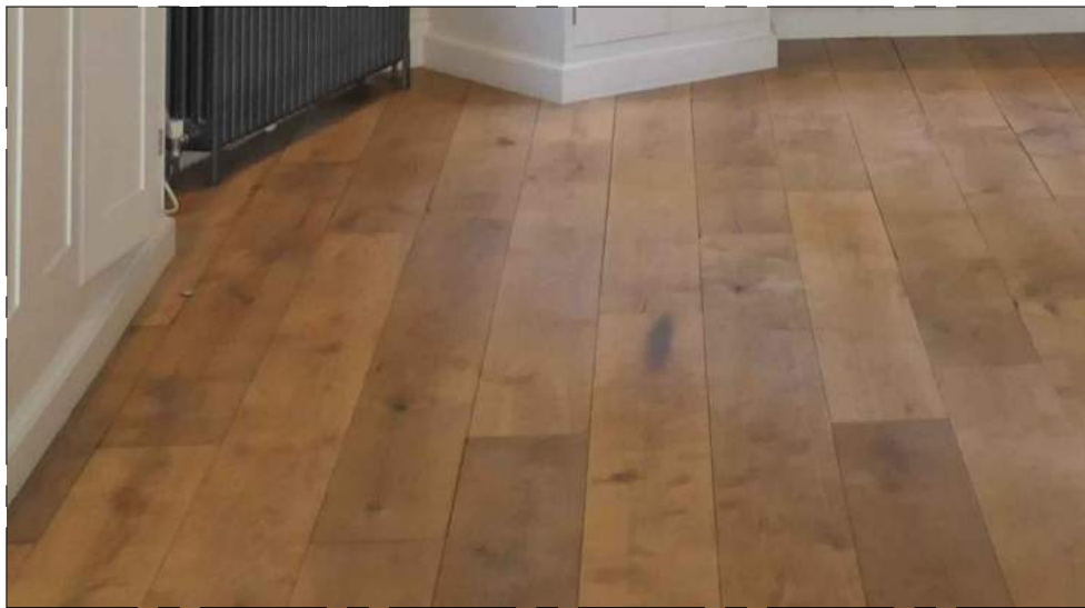
03 FLOORING 03 - TO BE REPLACED GROUND FLOOR - R04 KITCHEN
