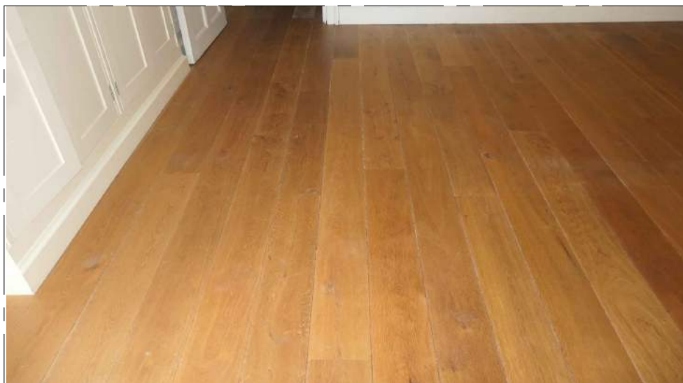
05 FLOORING 05 - TO BE REPLACED LOWER GROUND FLOOR - R09 BEDROOM 01
