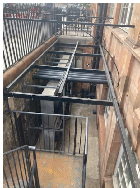
Existing building services plant within front basement area
