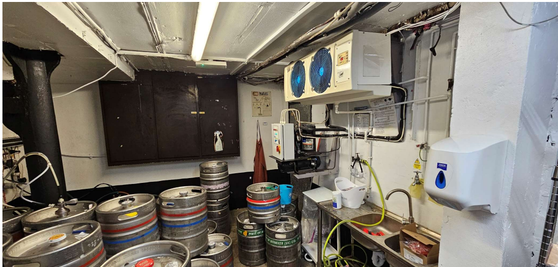
PUB CELLAR SHOWING EVAPORATOR UNIT LINKED TO FAN UNIT ON ROOF ABOVE
