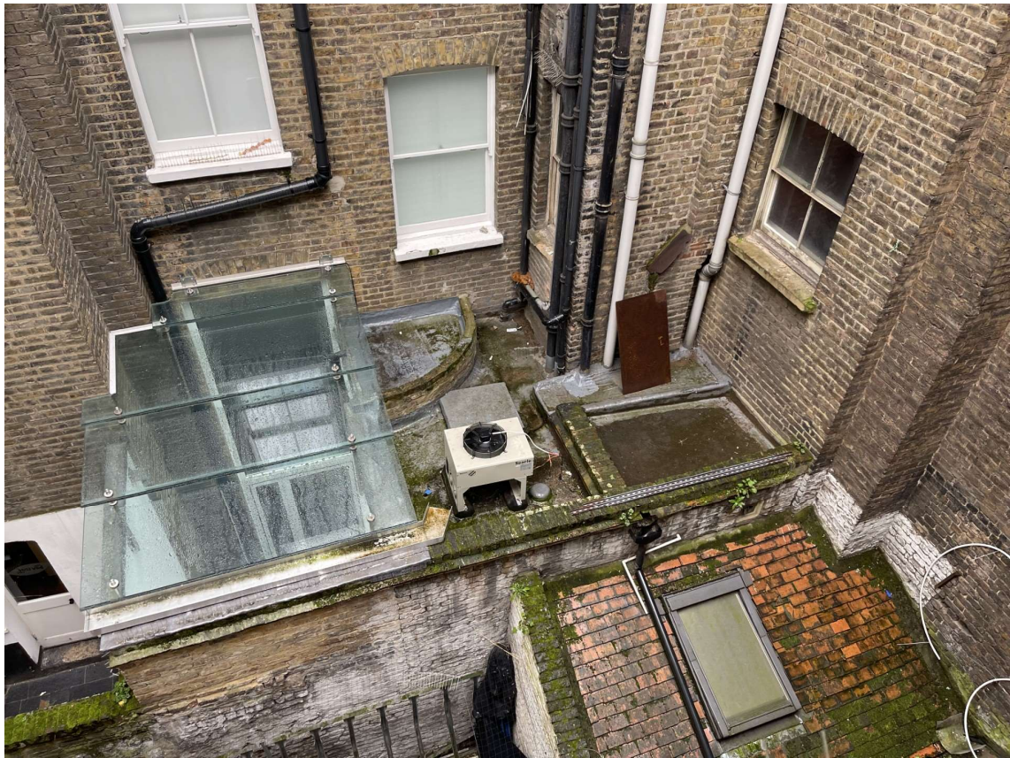
VIEW TO COURTYARD/ PUB CELLAR FLAT ROOF AND GLAZED CANOPY TO NO. 17
