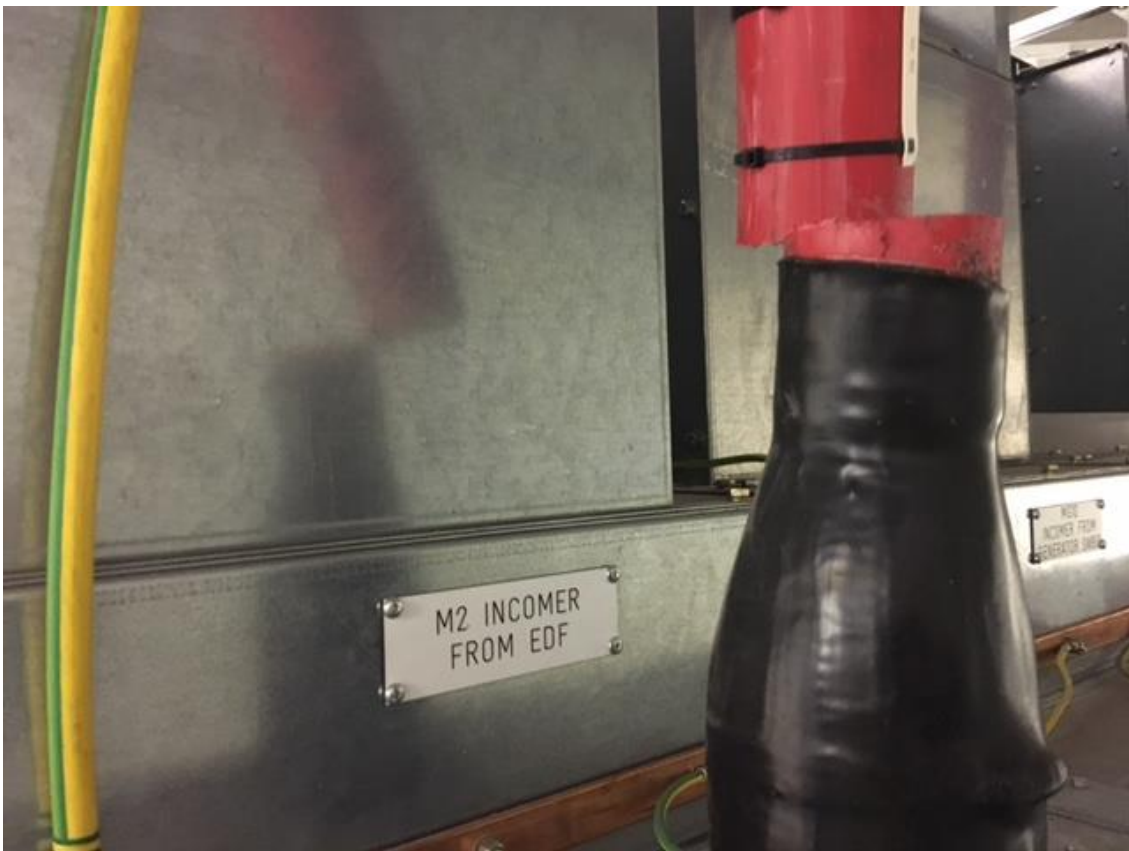
JP Morgan HV cables cut from within the two switch rooms.
