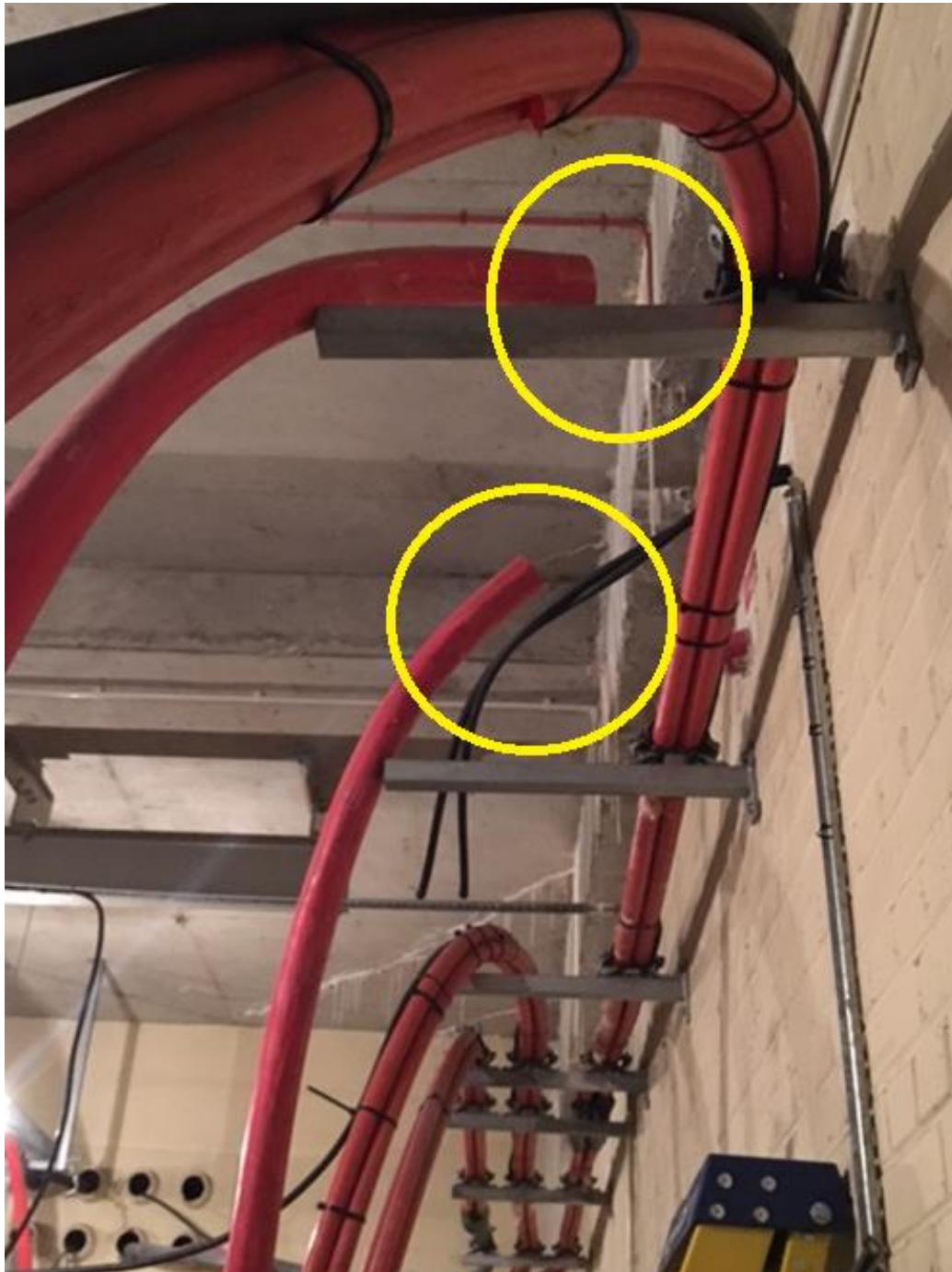
JP Morgan HV cables cut from within the UKPN switch room.
