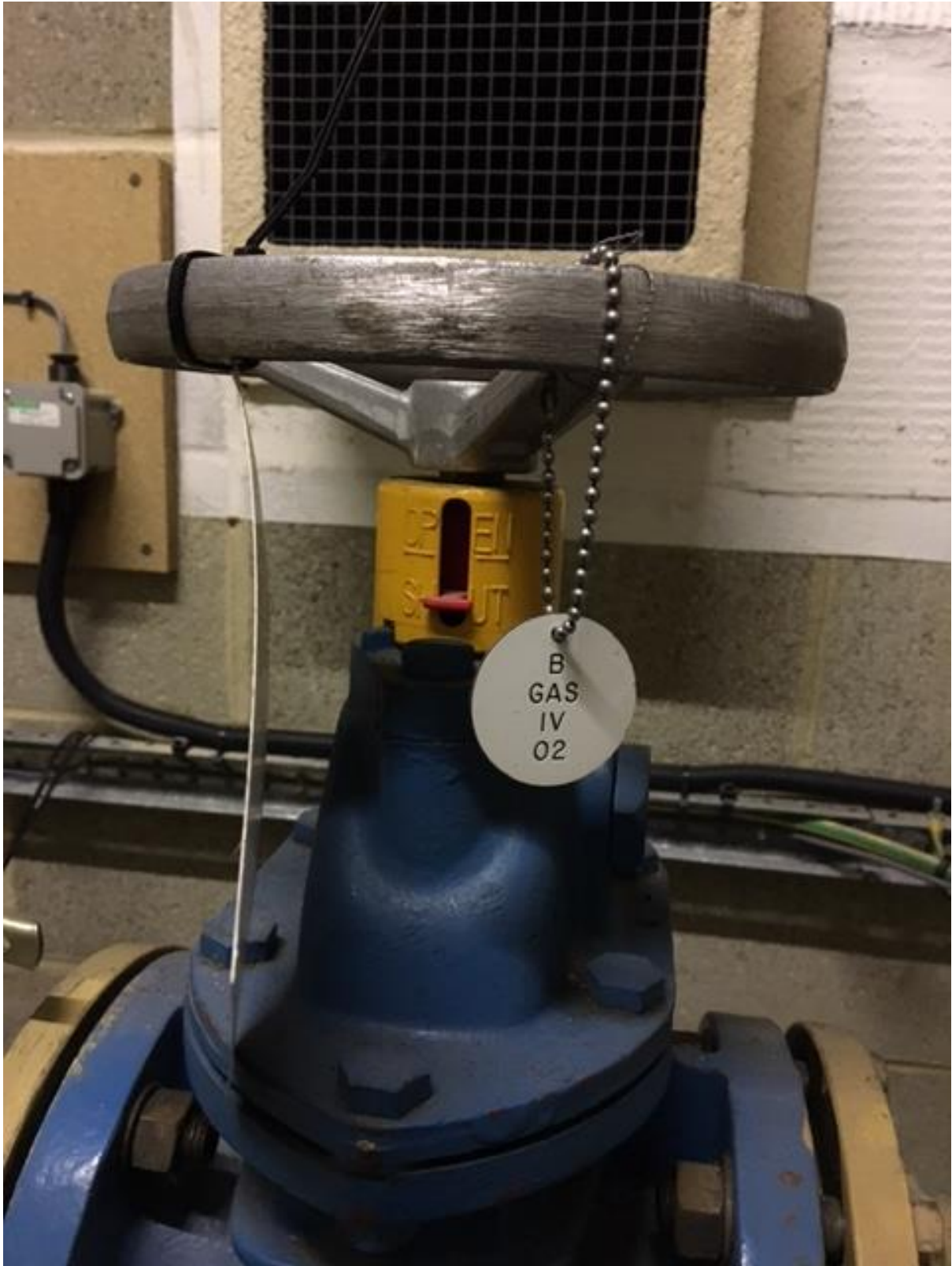
Gym Gas supply isolated
