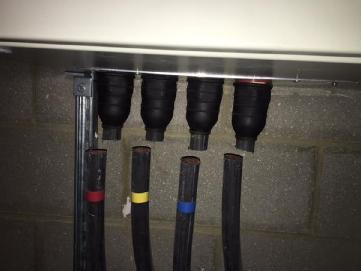
LV Supply cut from within the gym (Homes Place).
