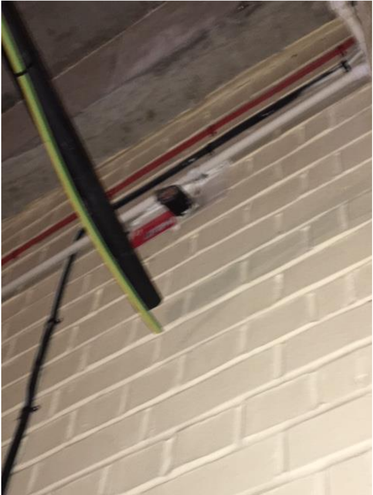
Service (unknown) supply cut within UKPN sub-station.
