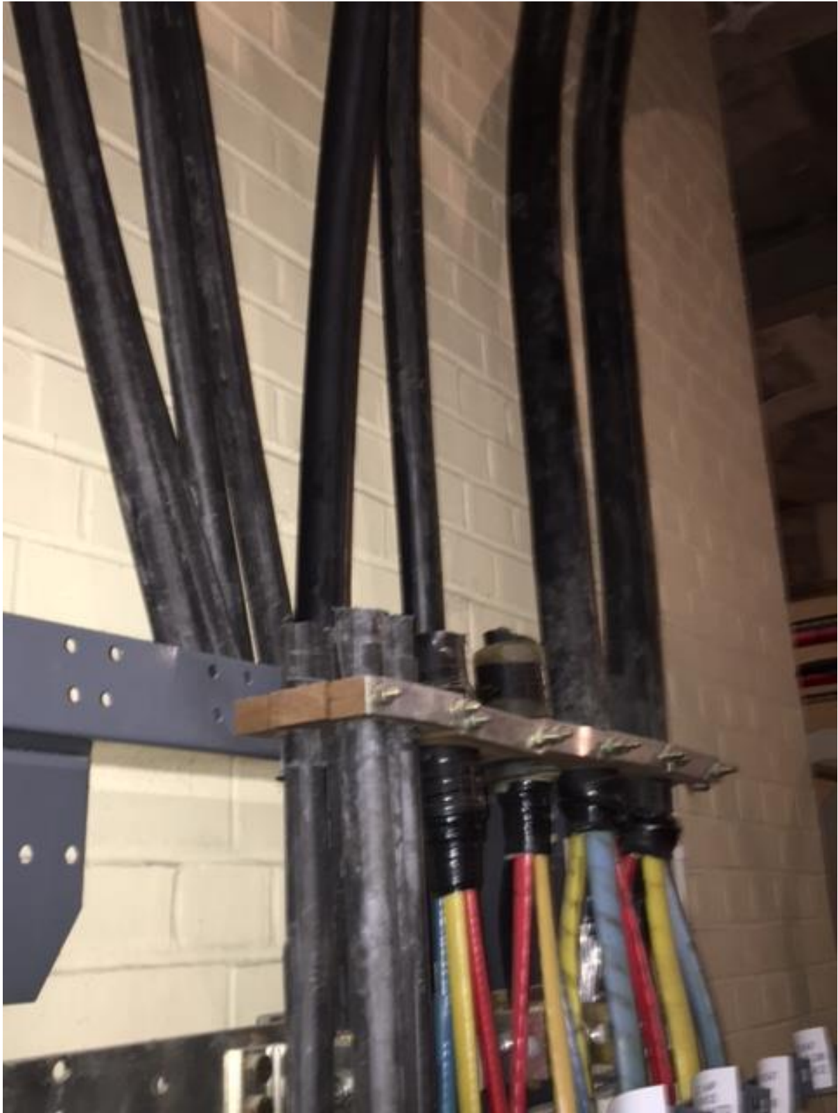
The Gym (Homes Place), Nursery (Kids Unlimited) and Service (Unknown) supplies cut within the UKPN sub-station.
