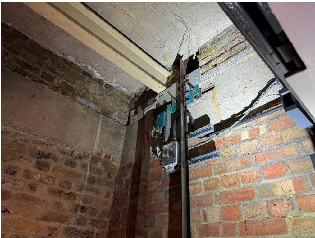
Figure 1: Picture inside lift shaft showing in-situ reinforced concrete cap spanning between masonry walls
