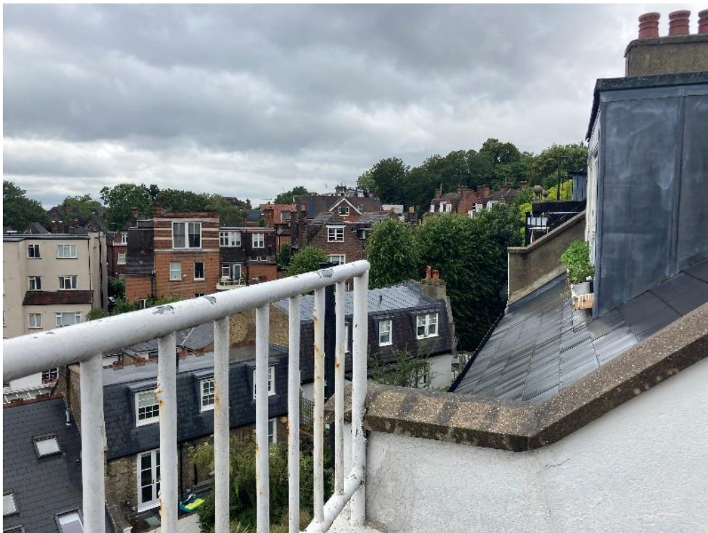
14. Site visit photograph, existing rear balcony railing.
