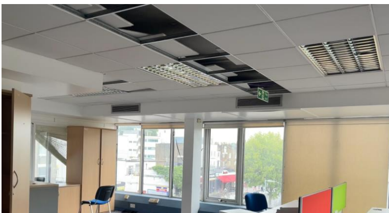
Figure 28 WEEE equipment (office)
