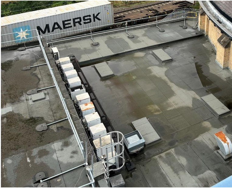
Figure 26 M&E equipment (workshop roof)
