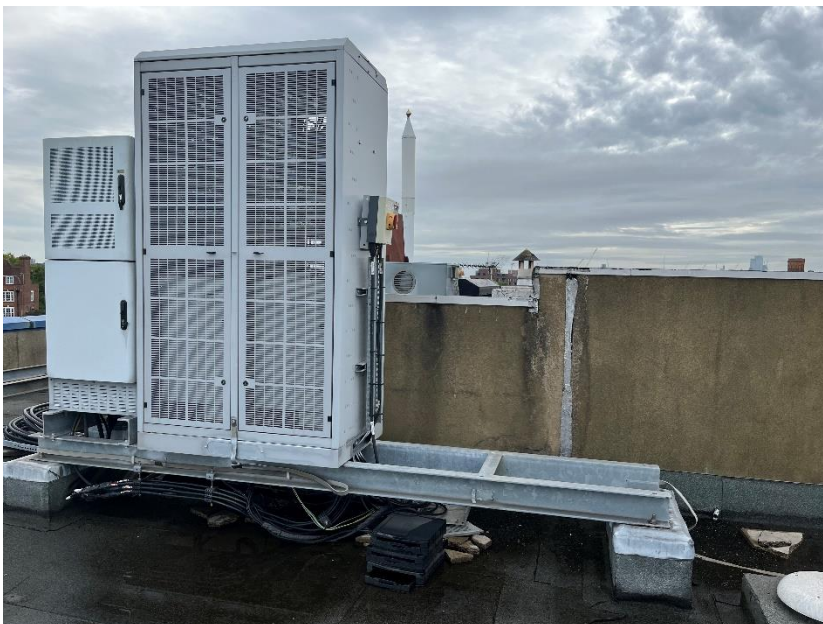
Figure 25 M&E equipment (office roof)
