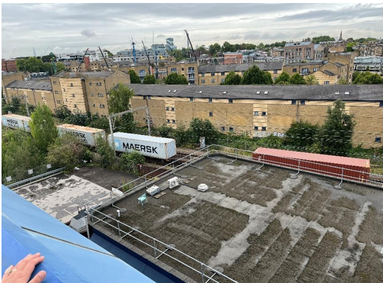
Figure 27 M&E equipment (workshop roof)
