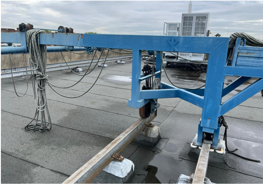
Figure 16 BMU unit and rails
