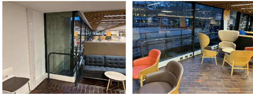
Figure 3 – Photos of the existing trunking that is proposed to be retained
