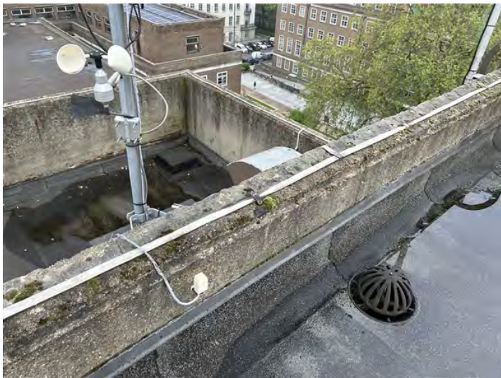
IMG_3894 (Area 3) Service Shaft Pooling water, perimeter lighting tape & rainwater outlet to be upgraded
