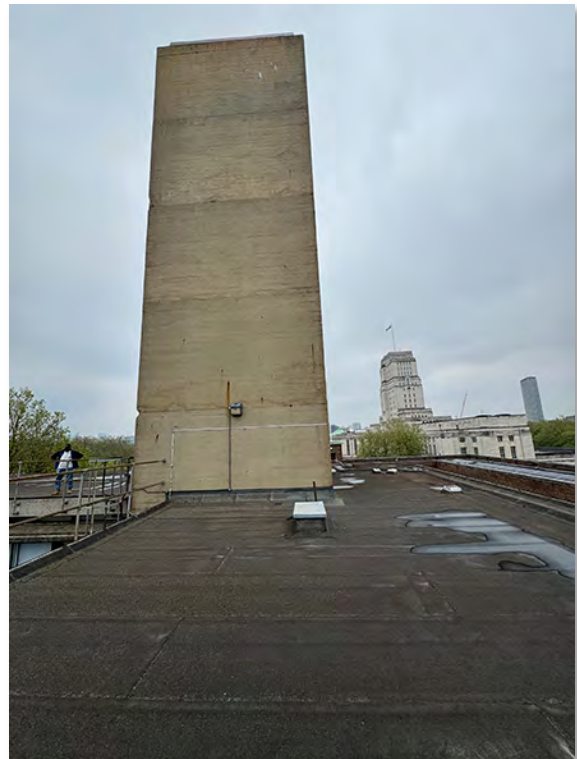
IMG_2736 (Area 2) Main Roof To the foreground, lead capped redundant ventilation housing proposed to be removed
