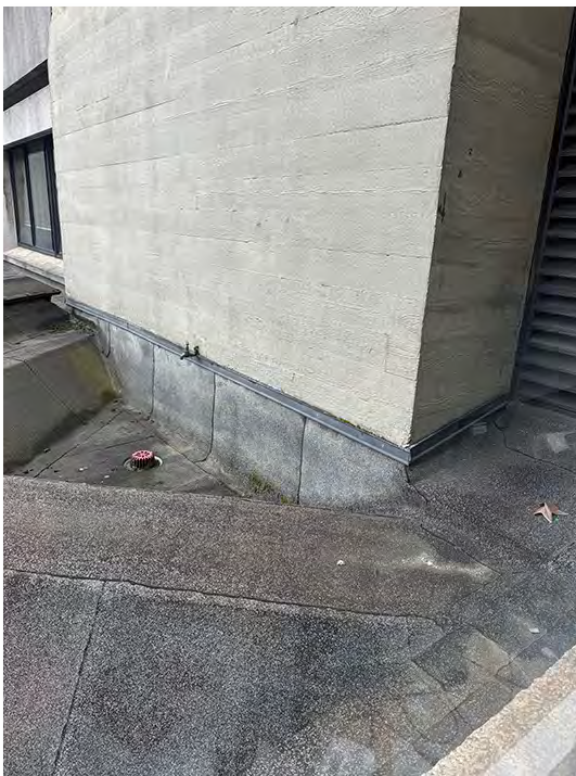
IMG_2770 (Area 1B) Library Roof Showing perimeter sunken well section of roof with drainage outlet
