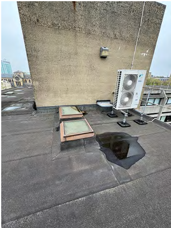
IMG_2735 (Area 2) Main Roof 2 x single glazed thermally inefficient roof lights proposed to be replaced
