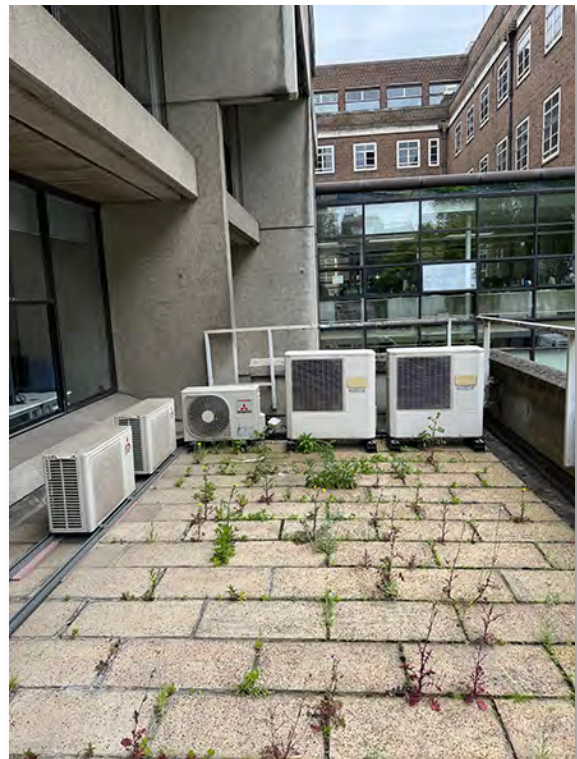
IMG_2901 (Area 7) AC plant to be retained
