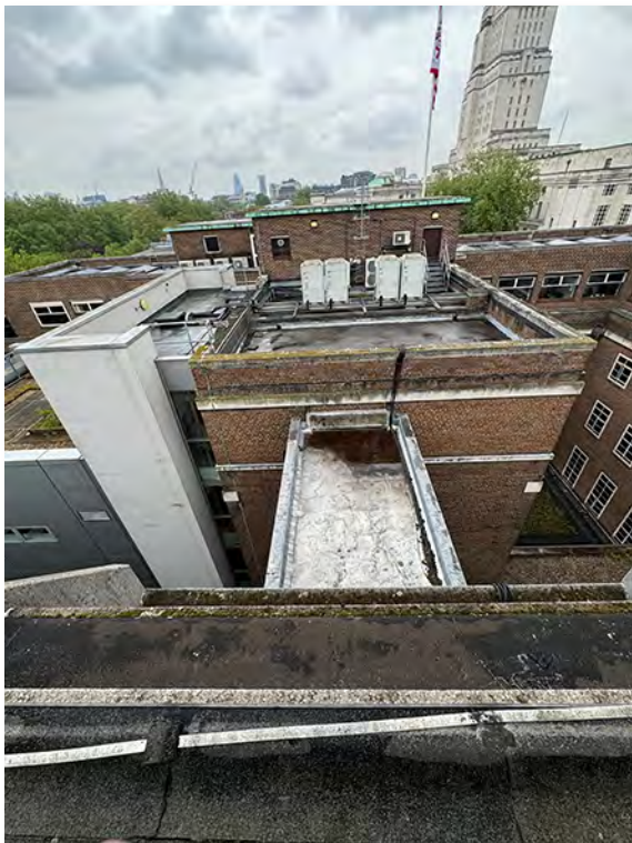
IMG_2921 (Area 9) Viewed from the Philips Building, with Link Bridge in the foreground
