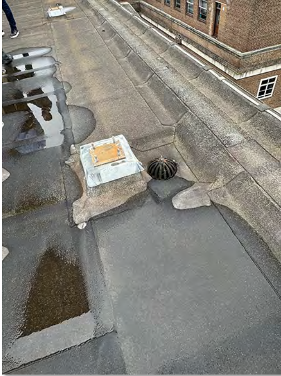
IMG_2739 (Area 2) Main Roof Raised perimeter kerb with formed concrete gutter, perimeter anchor blocks, proposed to be removed & rainwater outlet to be upgraded
