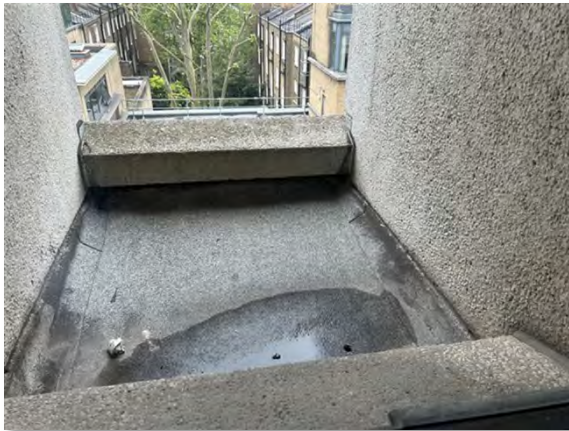
IMG_3915 (Area 4C) infill deck Example of 2 nd , 3 rd , 4 th & 5 th floor deck infill
