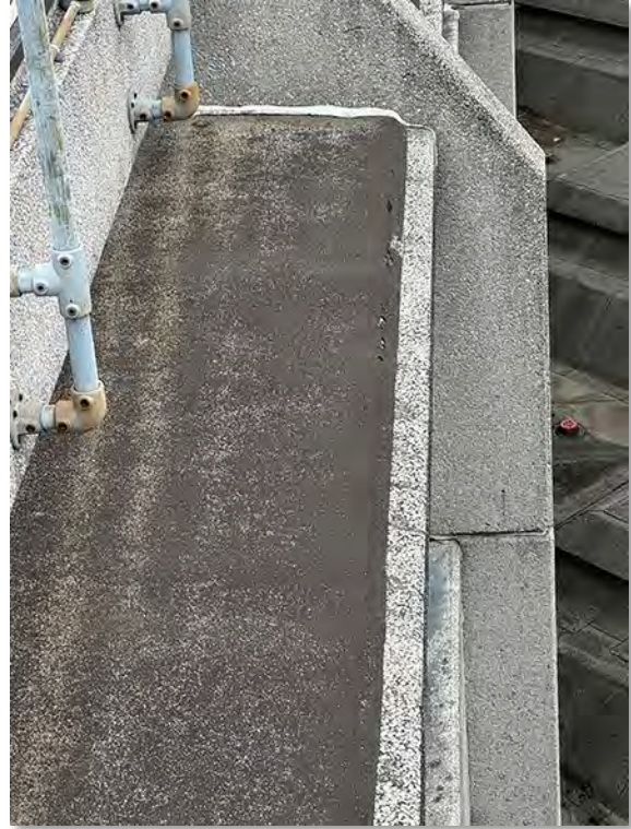
IMG_2763 (Area 4B) Canopies 5 th floor concrete perimeter inner window canopies with bitumen cap
