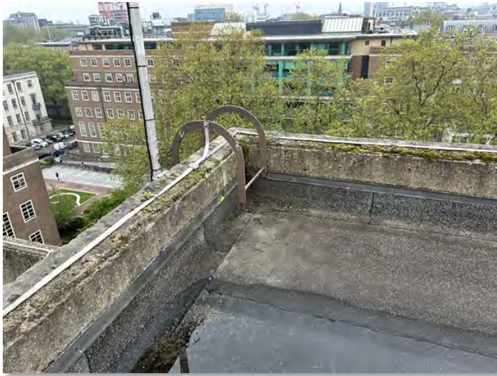
IMG_3896 (Area 3) Service Shaft Asphalt covering with upstand finished with galvanised capping strip.
