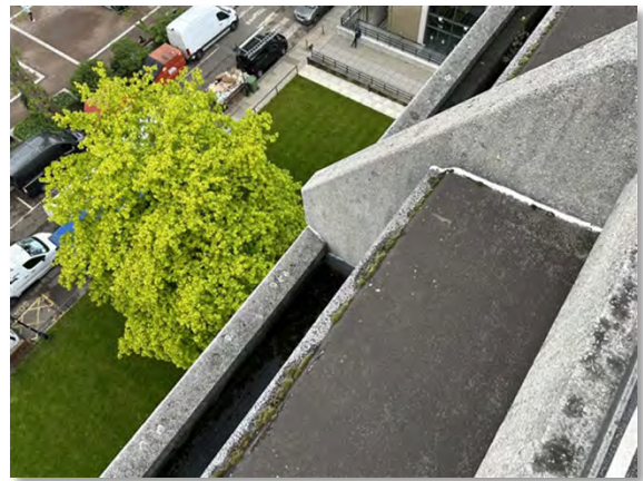
IMG_3913 (Area 4A) Canopies 5 th floor concrete perimeter inner window canopies with bitumen cap
