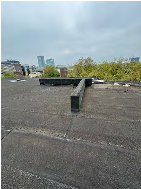
IMG_2751 (Area 2) Main Roof Concrete corner strap beam encased in waterproofing system
