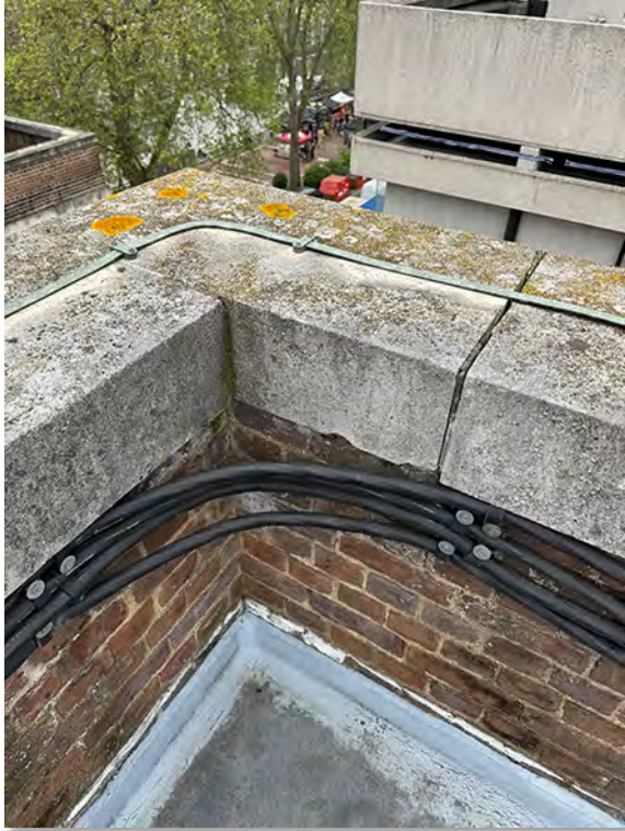
IMG_2725 (Area 9) Mortar joint failure between coping stones
