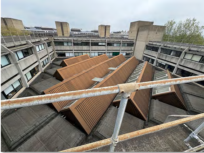
IMG_2729 (Area 1) Library Roof Showing the six rows of roof lights (Area A1) which are excluded from the proposed works.
