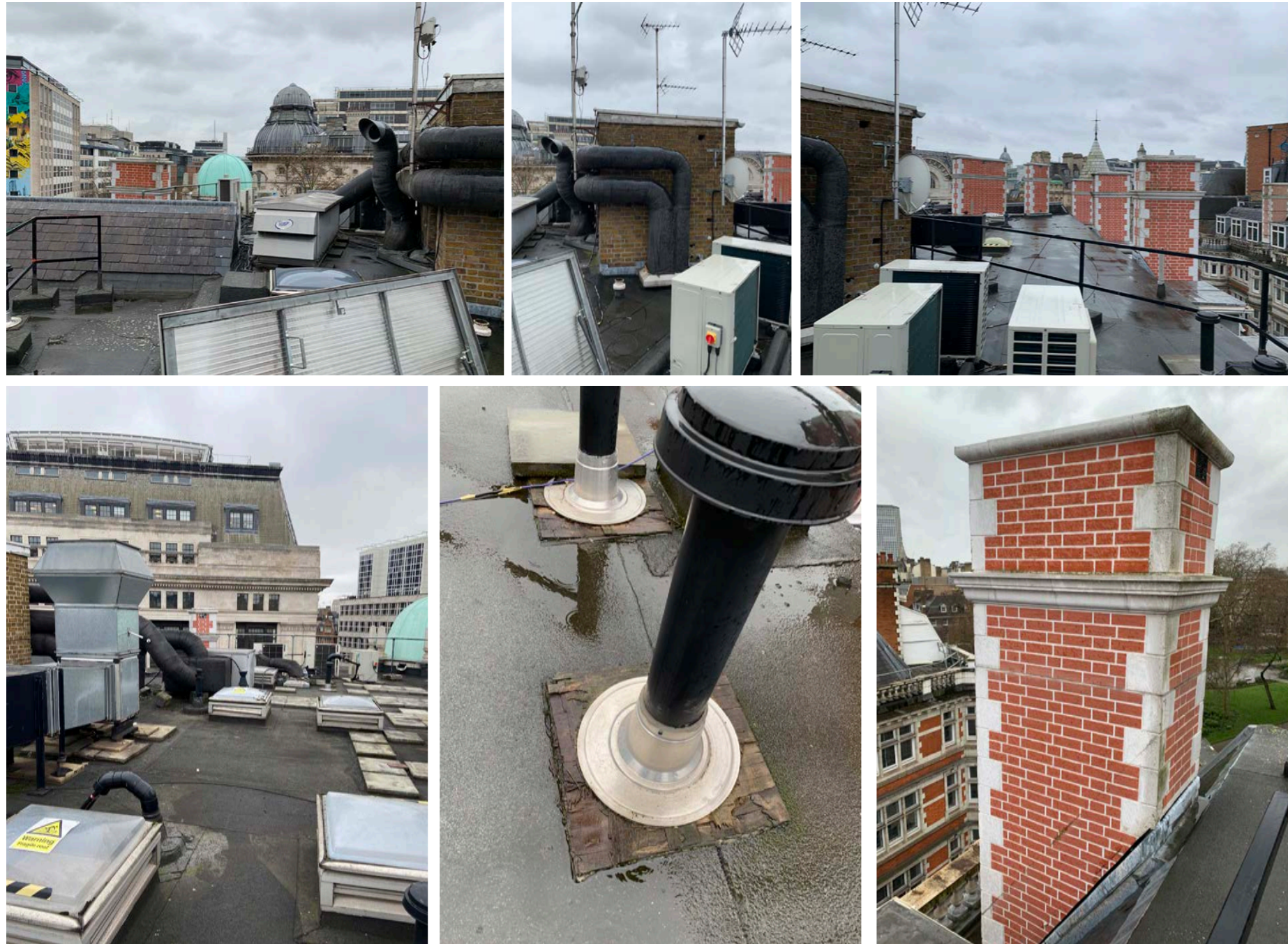
Existing roof top plant
